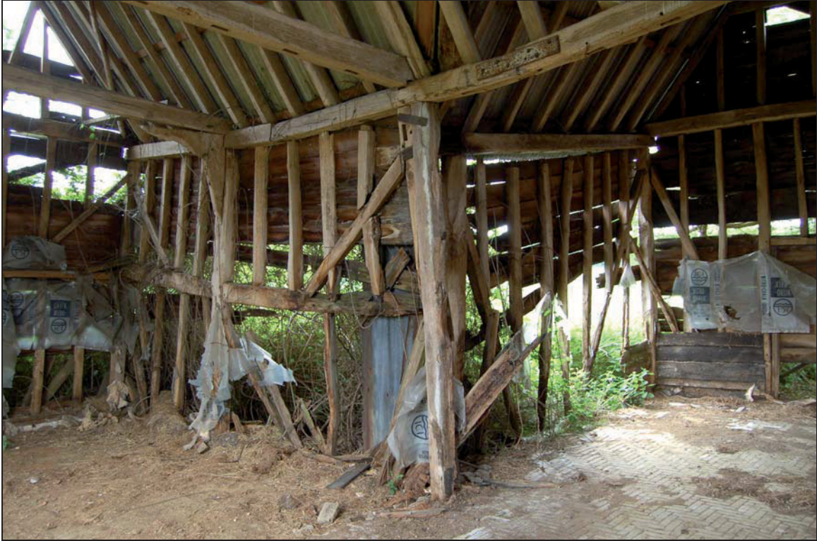
Plate 19 Dilapidated east end and porch in barn 3
