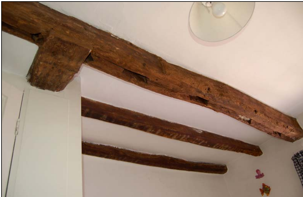
Plate 10 Detail of blocked mullion holes and pegged stud sockets to tie beam soffit
