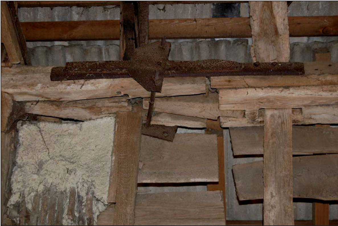
Plate 10 Crude un-halved bridle scarf joint inside barn 2 & remains of daub panel
