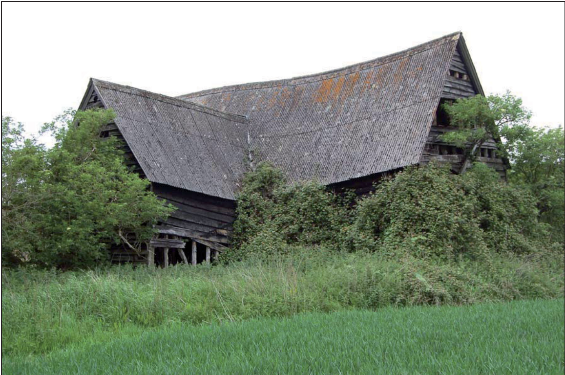
Plate 14 Collapsing barn 3 porch viewed from south-east
