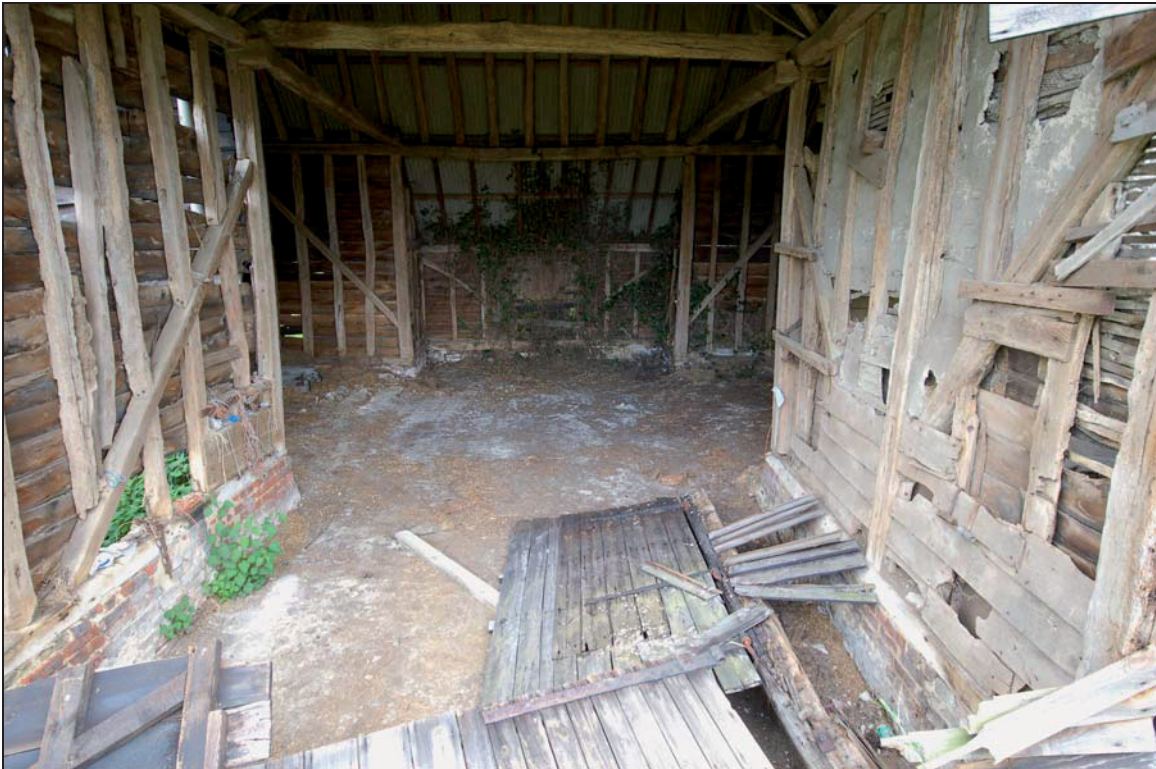
Plate 6 Collapsed cartdoors and plastered panels in barn 2 porch
