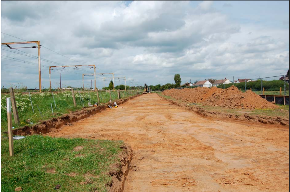
Plate 3. Northern end of Haul Road along east side of railway line, looking north
