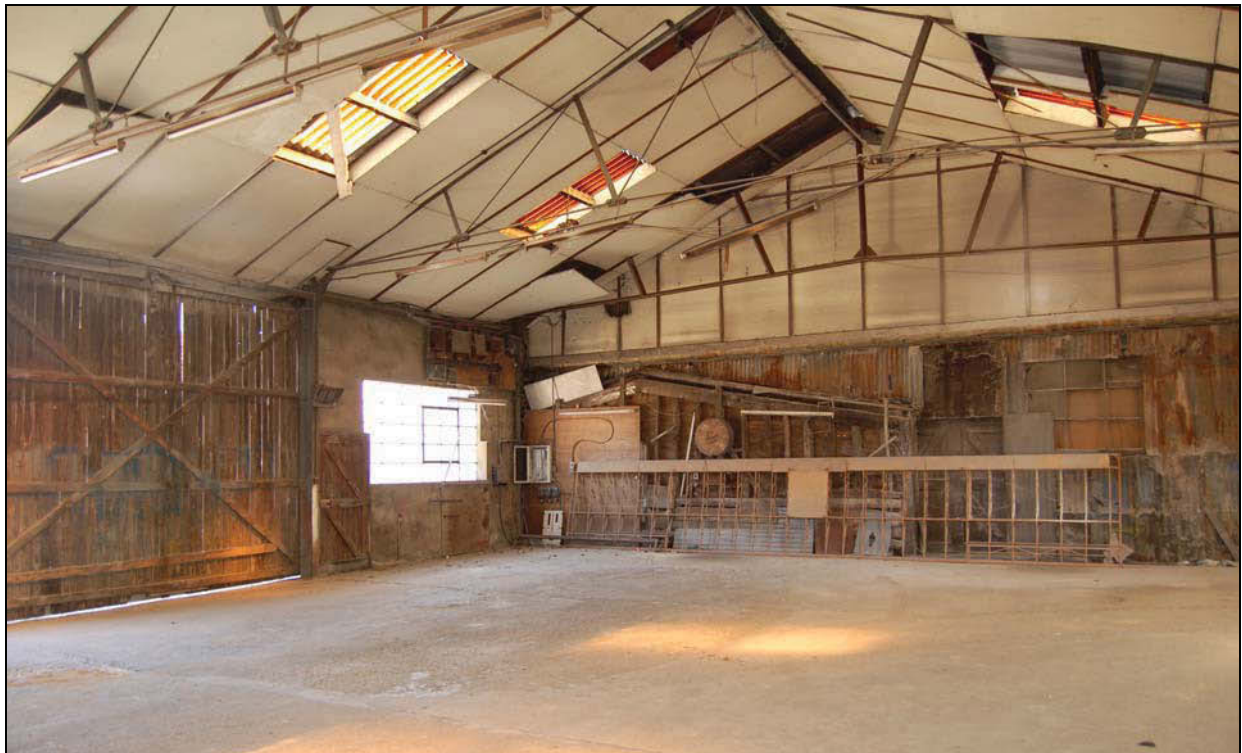
Plate 34 South wall of former cattle shed incorporated in south wall of Workshop 10
