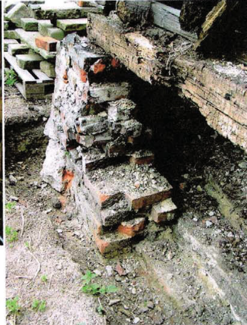
South-west corner showing plinth bearing on wall. This is the main cause of the plinth failure at this end.
