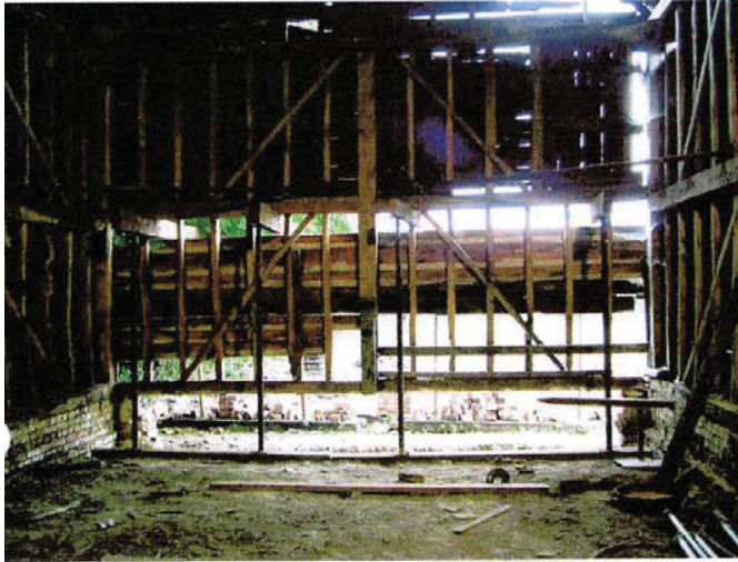
View to south end gable with plinth taken down and frame supported from mid rail.
