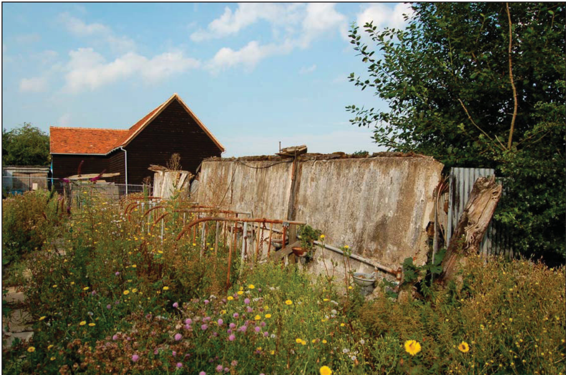
Plate 12 Derelict shelter shed viewed to west
