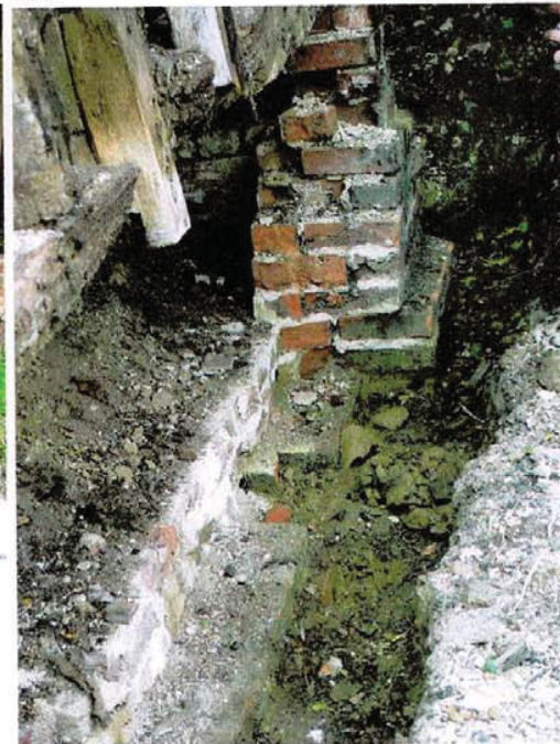
View to south corner showing plinth out of line with frame above.
