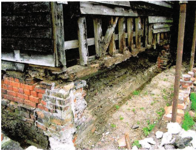
Outside view from the south-west showing full length of plinth wall and the badly eroded timber to sill plate and corner post.
