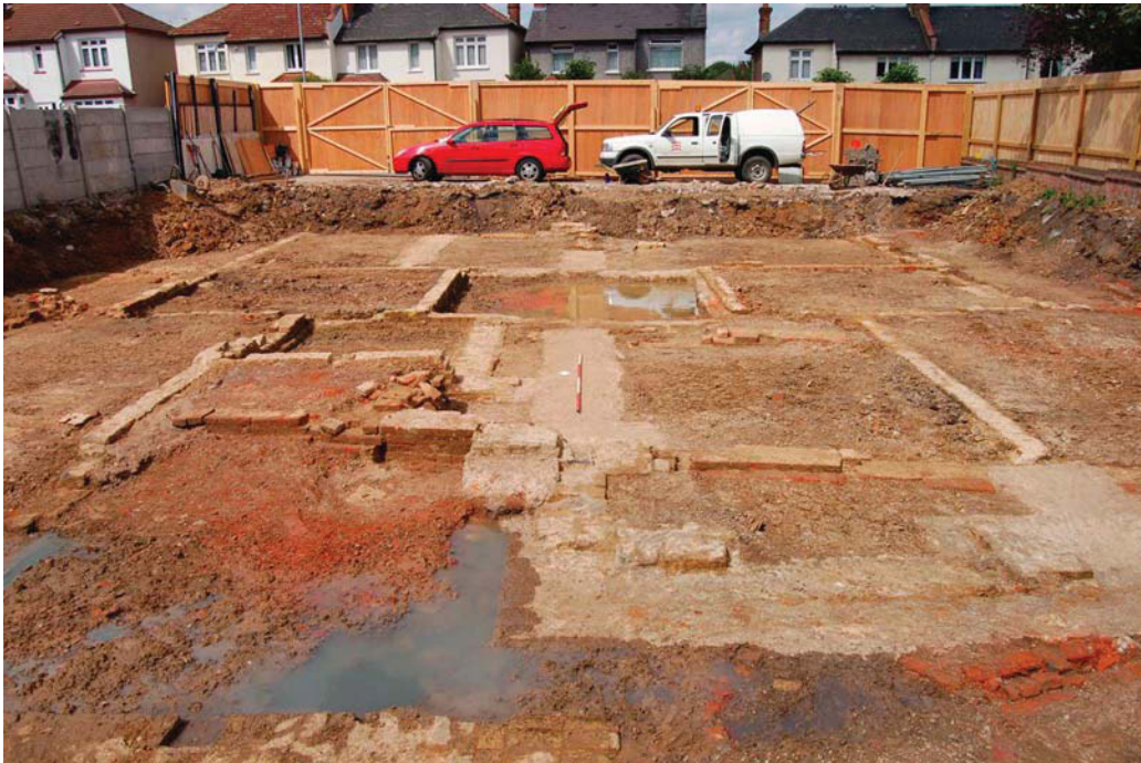
Plate 1. The site looking north, with remains of the late 16th/17th-century house overlain by modern foundations (2m scale)
