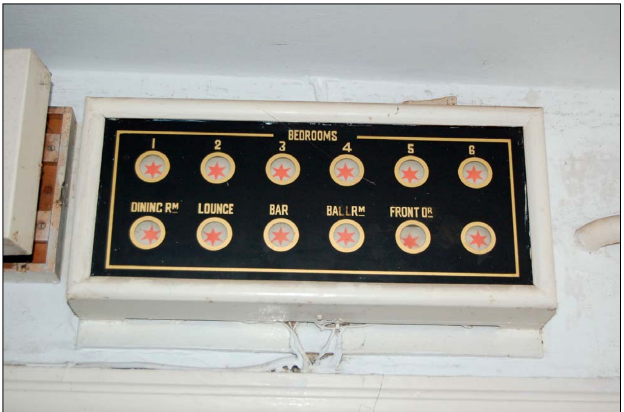
Plate 12 Service panel in breakfast room
