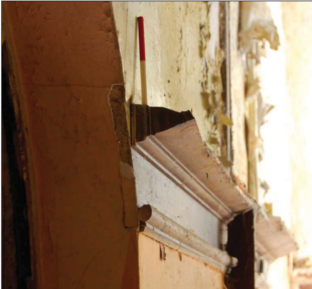
Plate 20 Arts and Crafts style picture rail in north-east corner of classroom (10cm scale)
