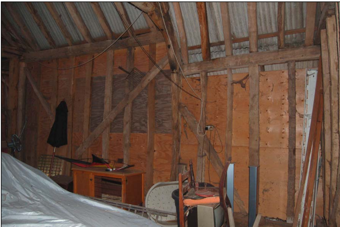
Plate 10 Intersection of barn and extension, showing different bracing forms on south wall
