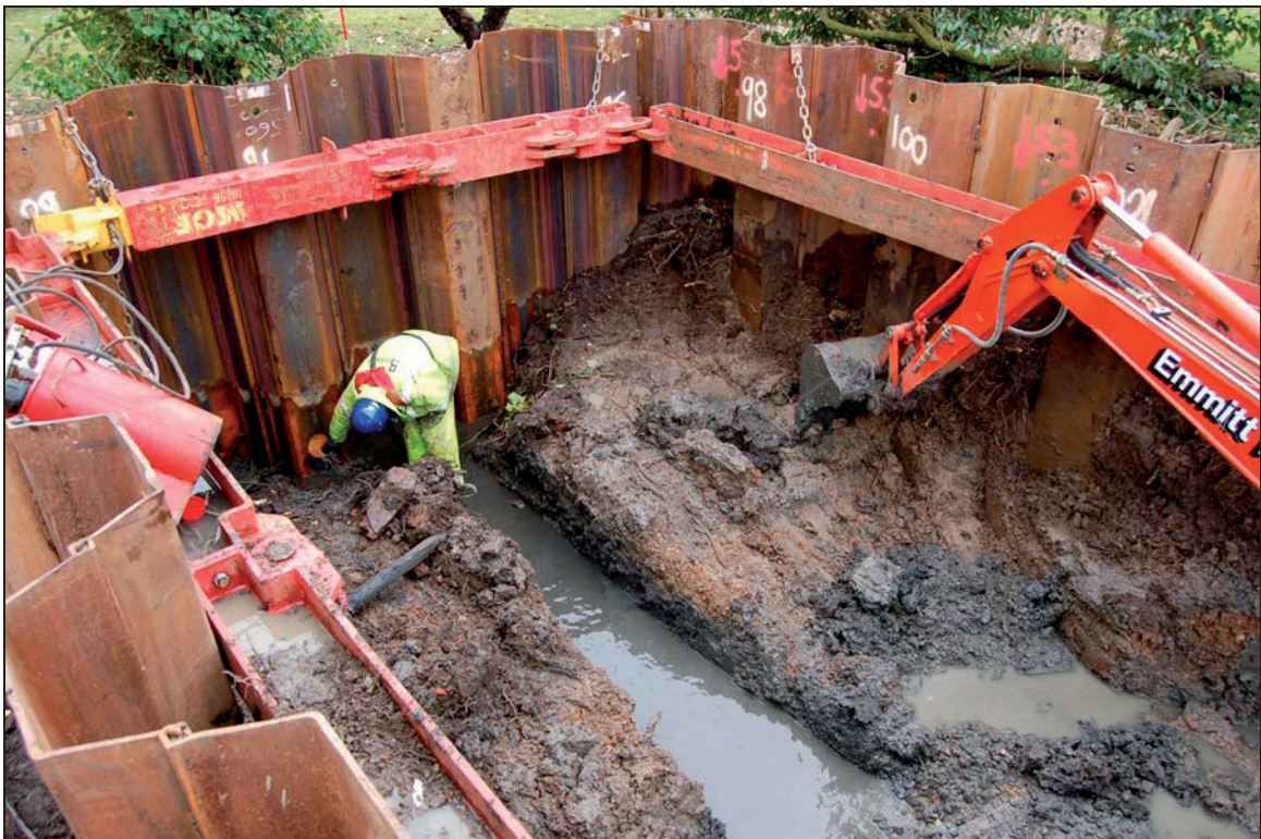
Plate 2 Undisturbed soil deposits underneath bank at south-east end
