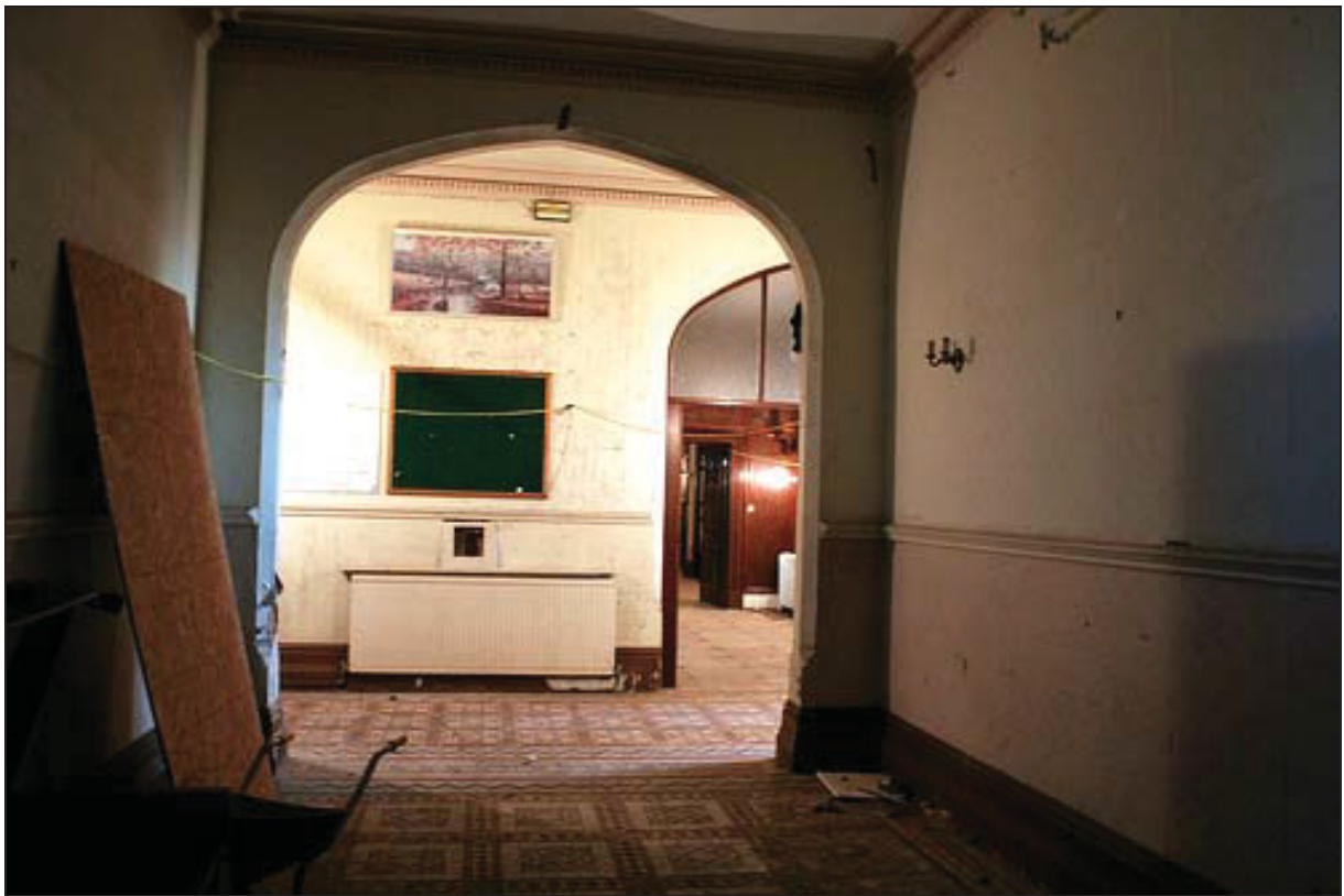
Plate 12 View from entrance hall to lobby in 2007 (Derelict buildings.co.uk)
