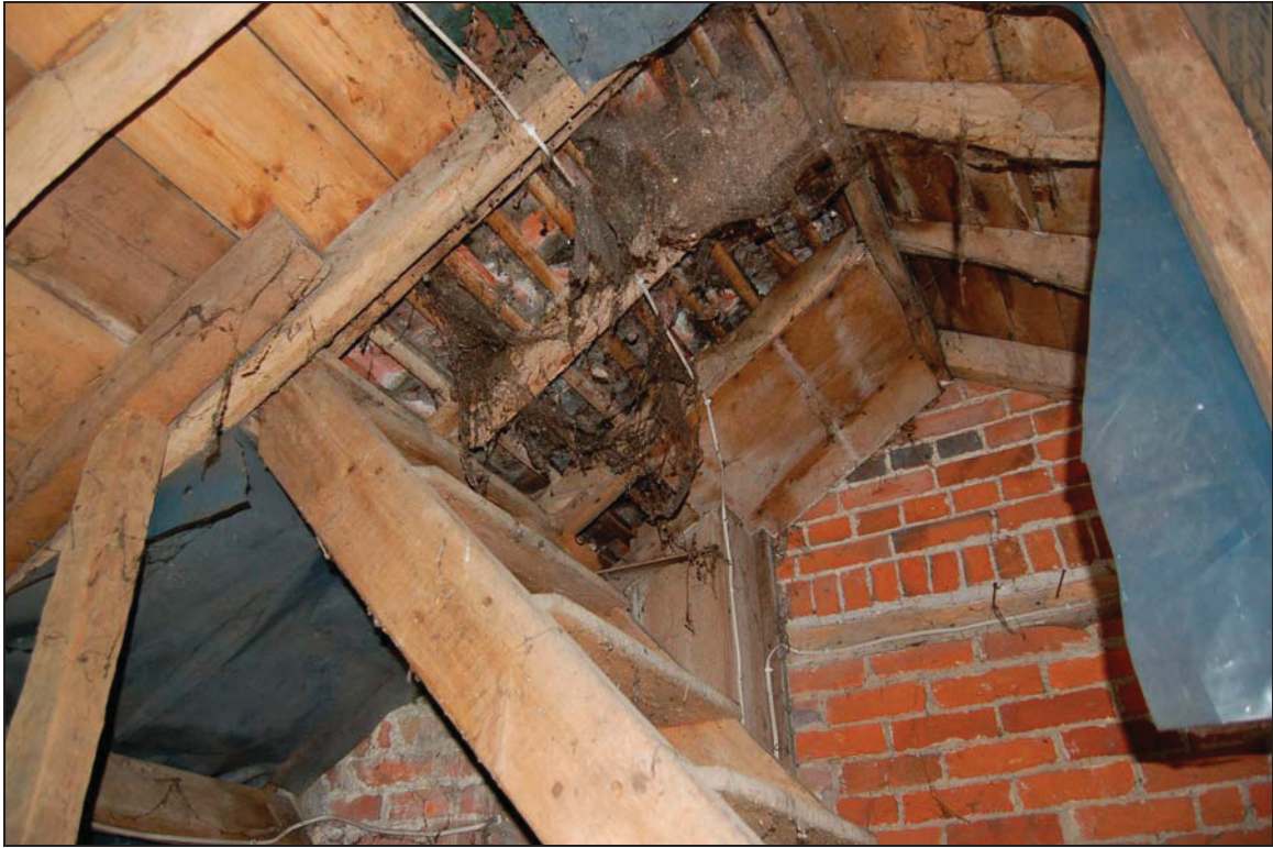
Plate 41 Blocked roof access in feedstore
