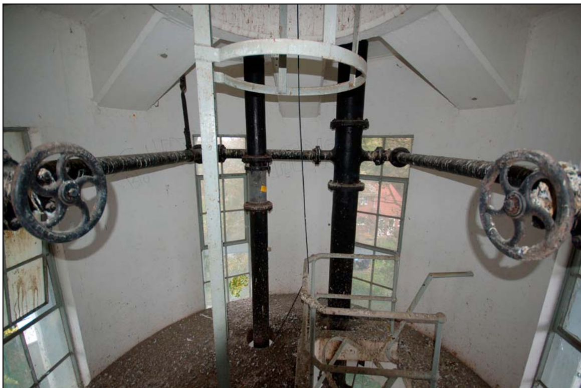
Plate 8 Delivery and washout/overflow pipes in valve room (level 2)
