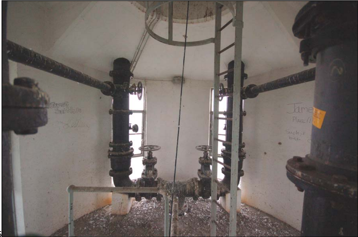
Plate 7 Inlet and outlet pipes in valve room (level 2)
