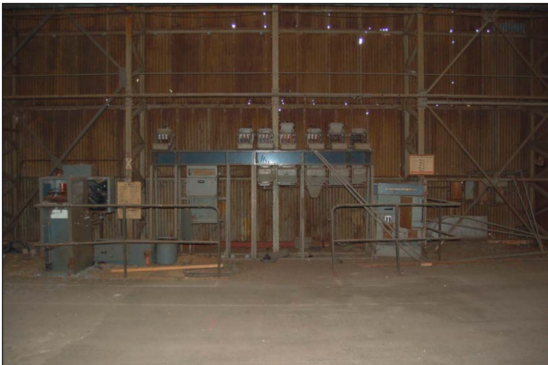
Plate 8 Electricity sub-station/switch box
