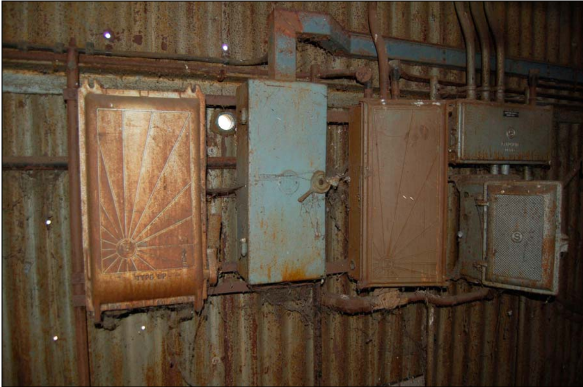
Plate 9 1940s Fuse boxes
