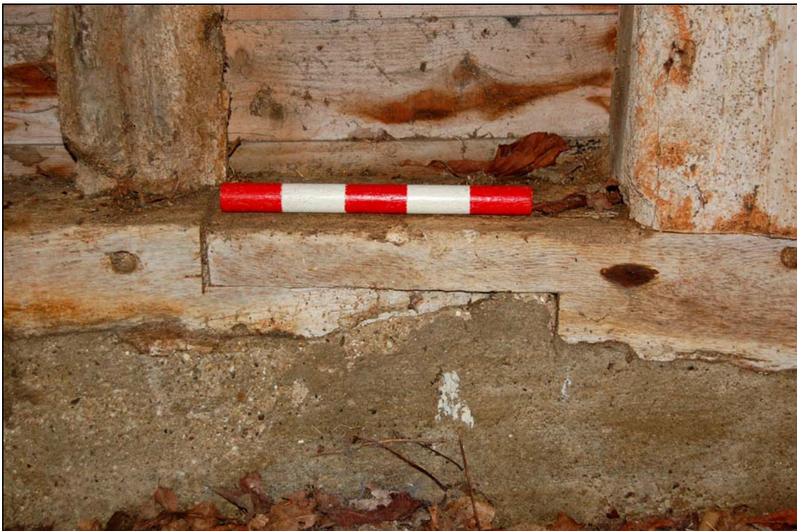
Plate 8 Typical lapped scarf joint in sill plate
