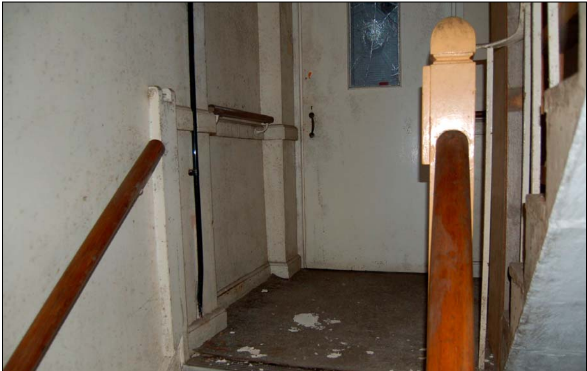
Plate 34 Remains of stair guard on first floor landing
