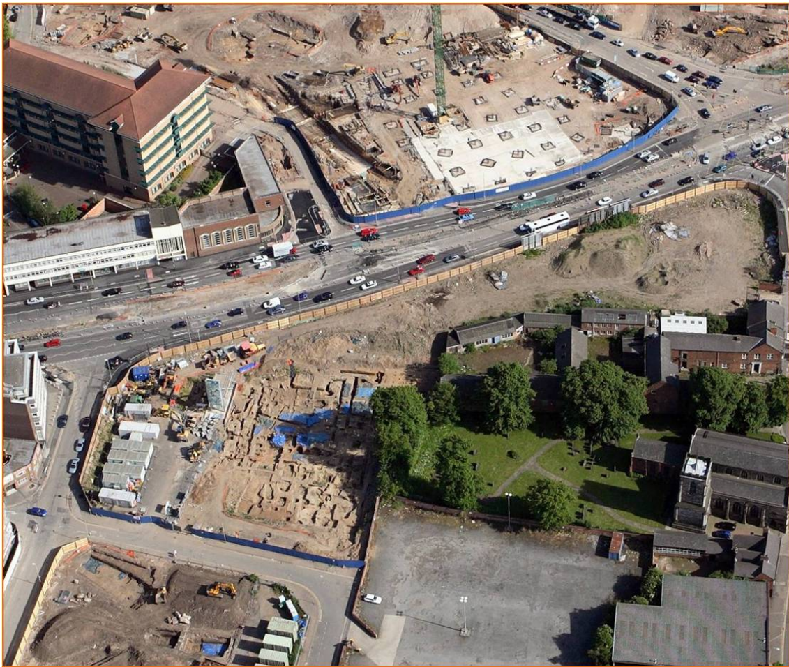
Figure 2 Aerial photograph of the site under excavation, with the Burgess Street evaluation in progress. View south.
