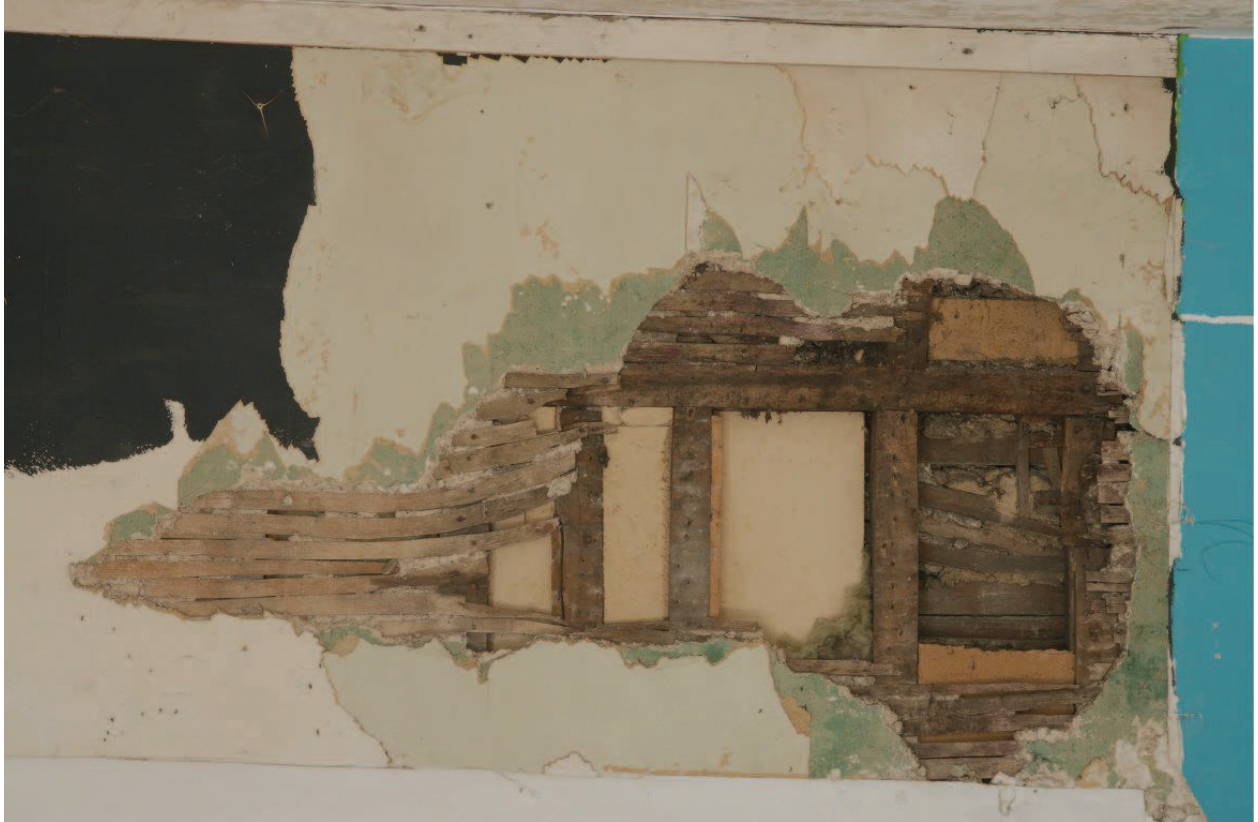
Plate 08 - Detail of exposed studwork in W elevation of living room, looking W
