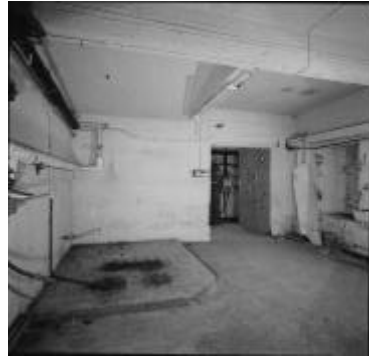
8 Plant room: general shot facing east
