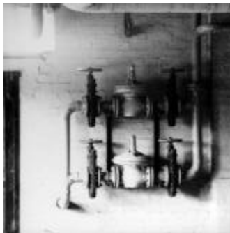
4 Boiler House: gas inlet pipes
