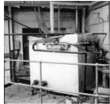
6 Boiler House: water tank
