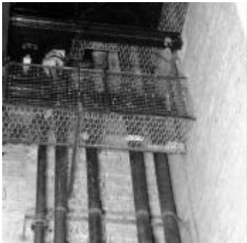
10 Water Tower: south-east pipework from mezzanine
