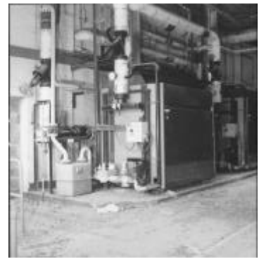
3 Boiler House: gas-fired boiler
