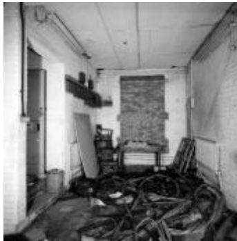
4 Engineer's Block: switch room facing south
