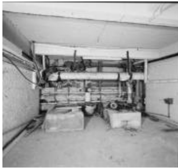
7 Plant room: general shot facing west
