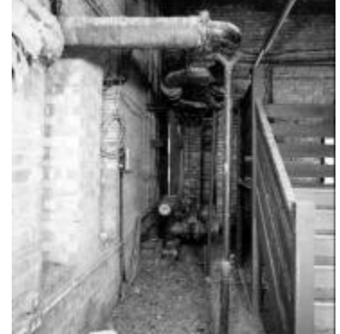
3 Water Tower: pipework in south-east corner
