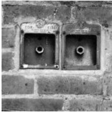
1 Engineer's Block: south elevation fire alarm detail
