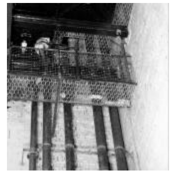
9 Water Tower: south-east pipework from mezzanine
