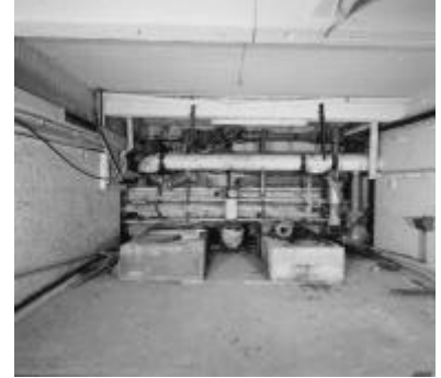
9 Plant room: general shot facing west
