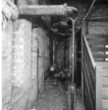
2 Water Tower: pipework in south-east corner
