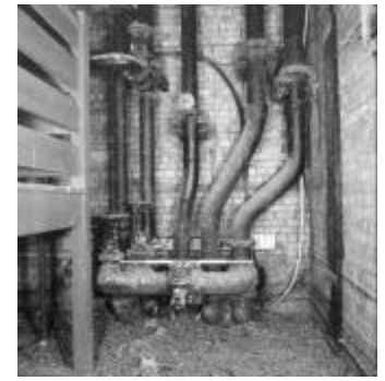
9 Water Tower: pipework in the south-east corner
