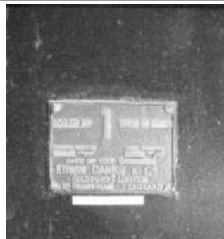
8 Boiler House: boiler plaque
