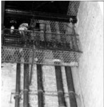
7 Water Tower: south-east pipework from mezzanine
