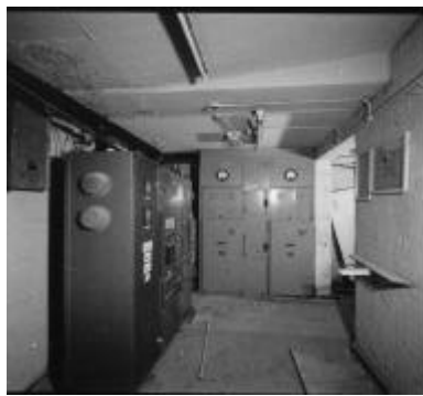
5 Switch Room: general shot facing south
