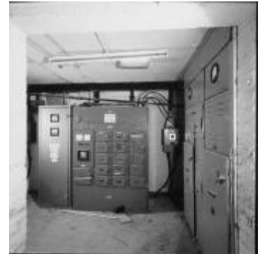
6 Switch Room: plant
