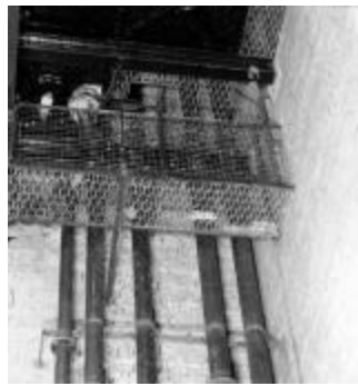
8 Water Tower: south-east pipework from mezzanine
