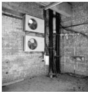
11 Water Tower: pipework in the north-east corner
