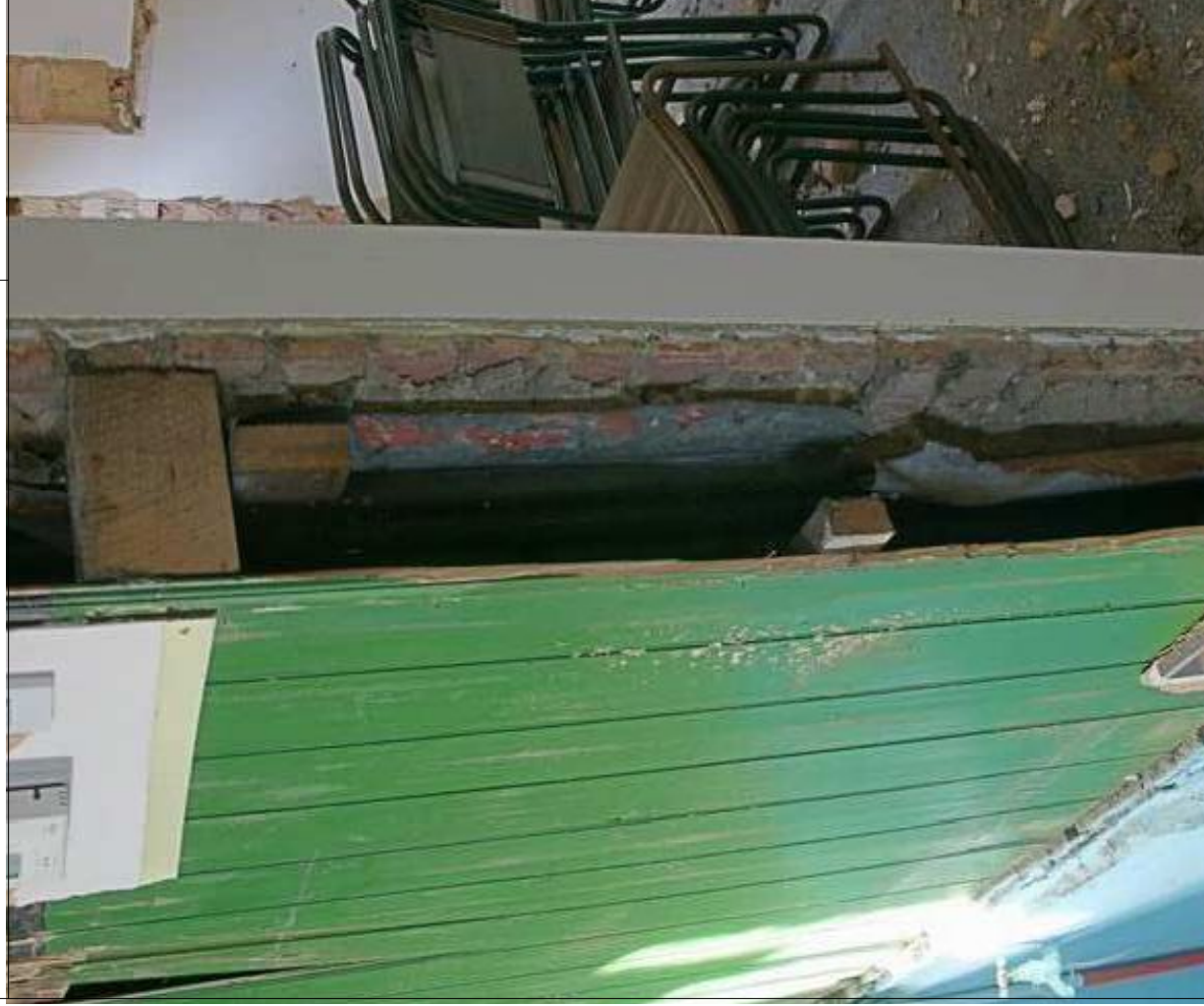
Plate 15: Section through north-west gable wall showing cut battens and interior and exterior wall facings
