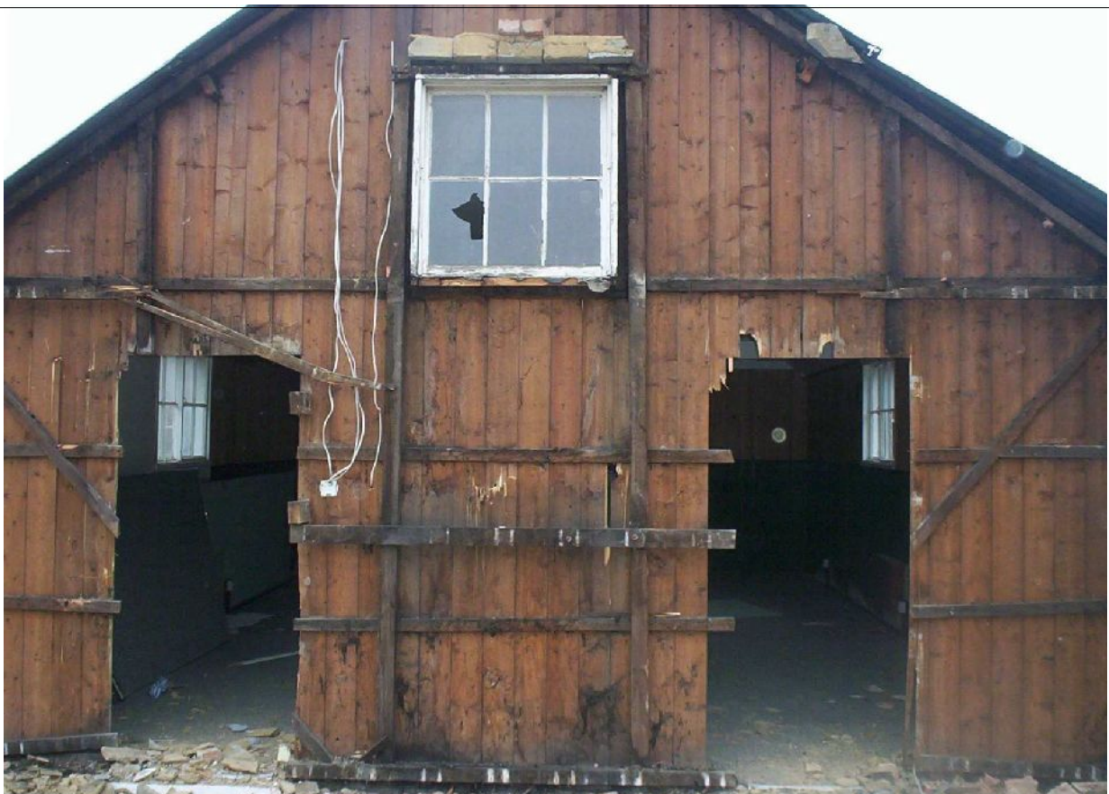
Plate 14: North-west gable end of The Gospel Hall after demolition of the extension
