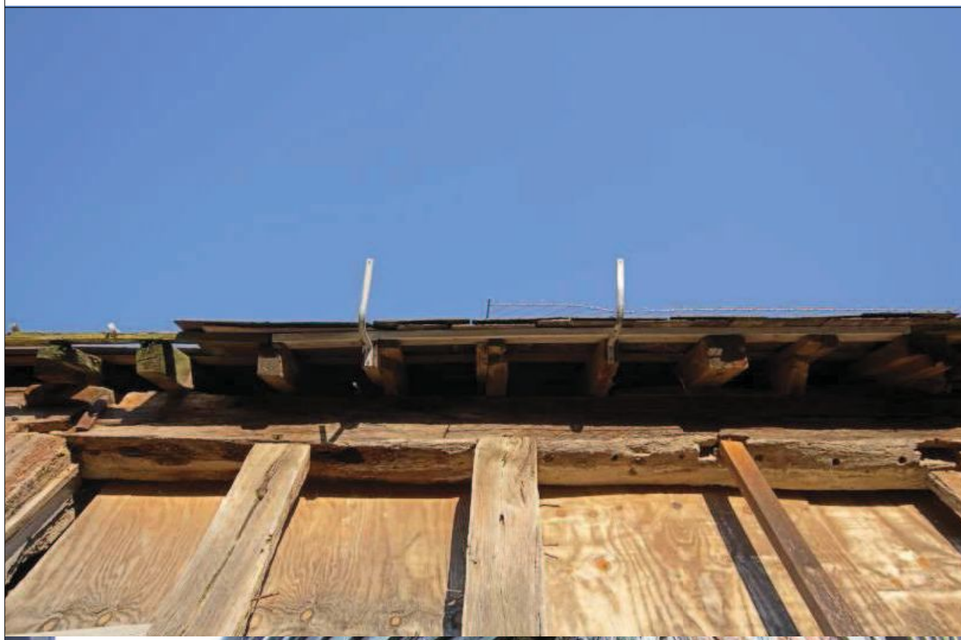
Plate 10: Detail shot, underside of wall plate in Bay 2, west elevation, showing dowel holes
