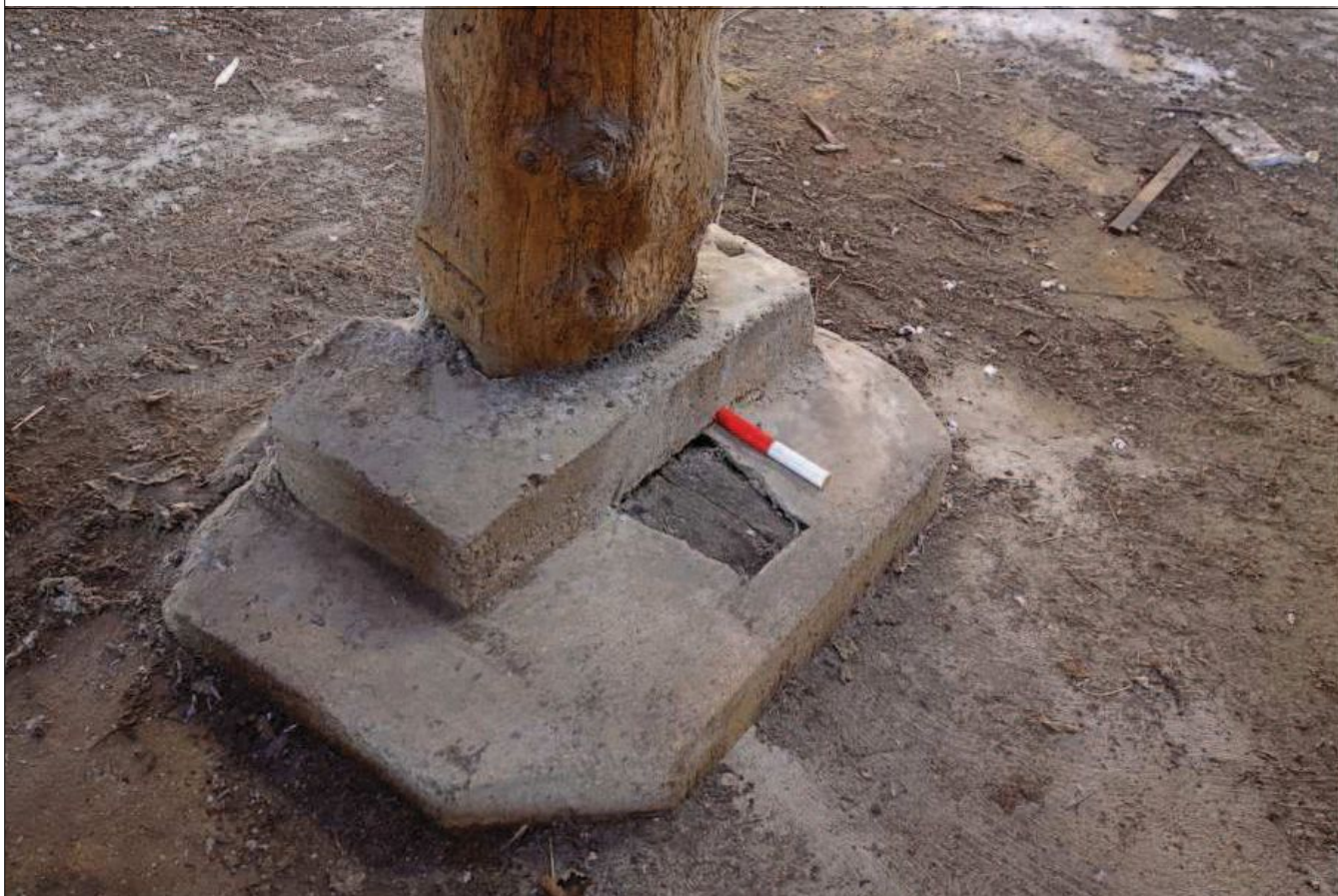
Plate 22: Detail of concrete pad below arcade post and remains of peninsular sill
