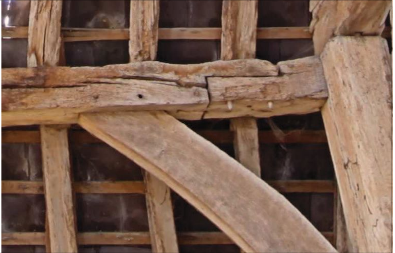
Plate 17: Edge halved and bridled scarf joint to W arcade plate, Bay 7
