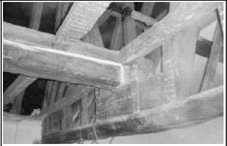
DP6: Annexe, main room, junction of tie-beam with joist-beam
