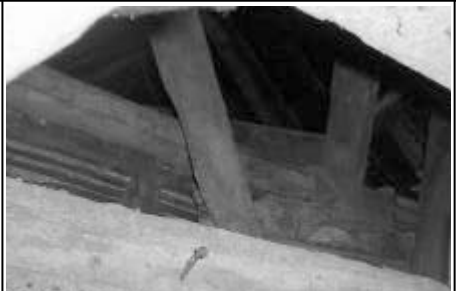
DP12: Annexe, ceiling structure at junction former kitchen & main room looking NW
