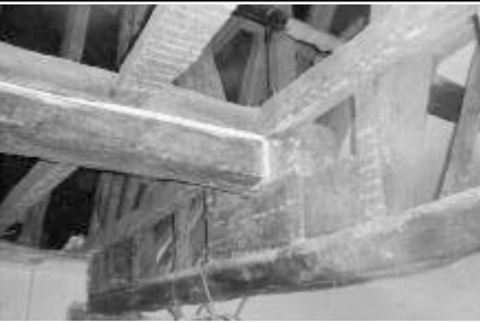
DP5: Annexe, main room, junction of tie-beam with joist-beam
