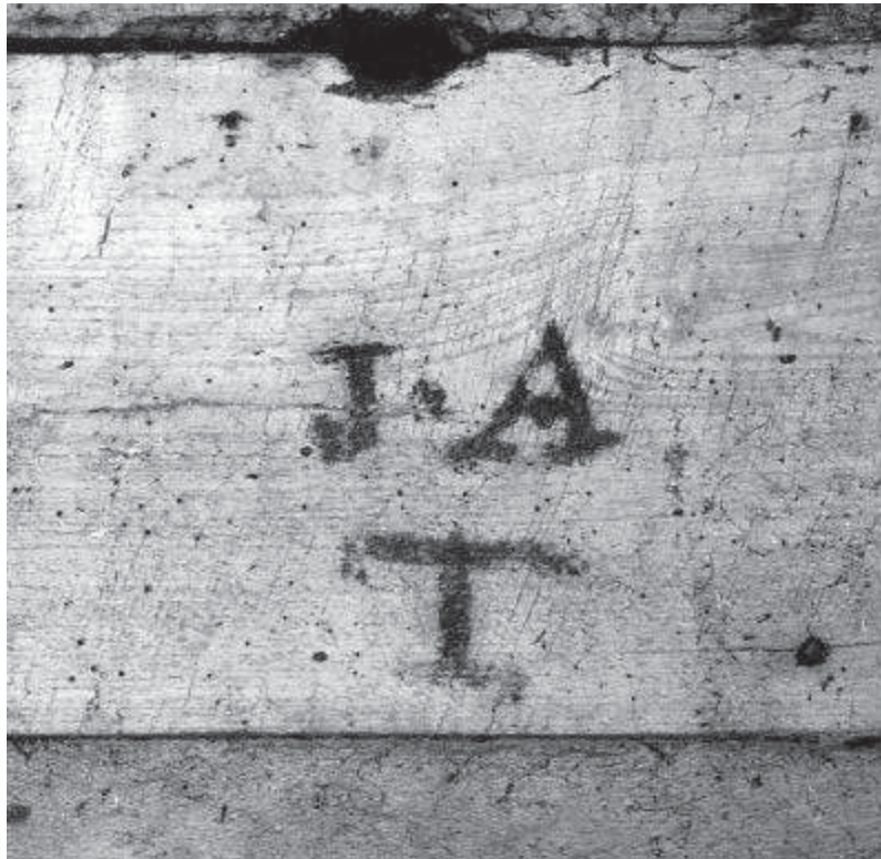
Graffiti on the west elevation of the porch
