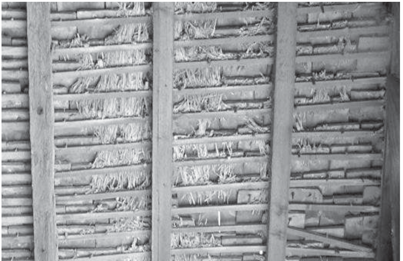
Plate 6: Straw 'torching' in barn roof
