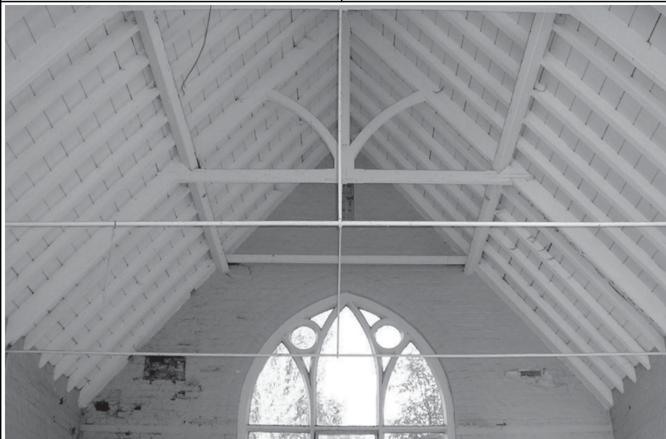
Plate 16: Building 2, classroom ceiling
