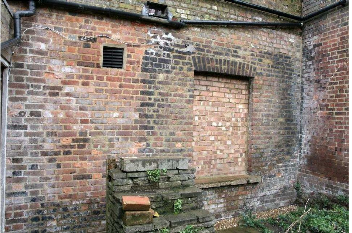
Plate 05 - Rear exterior elevation of No2 showing blocked window opening
