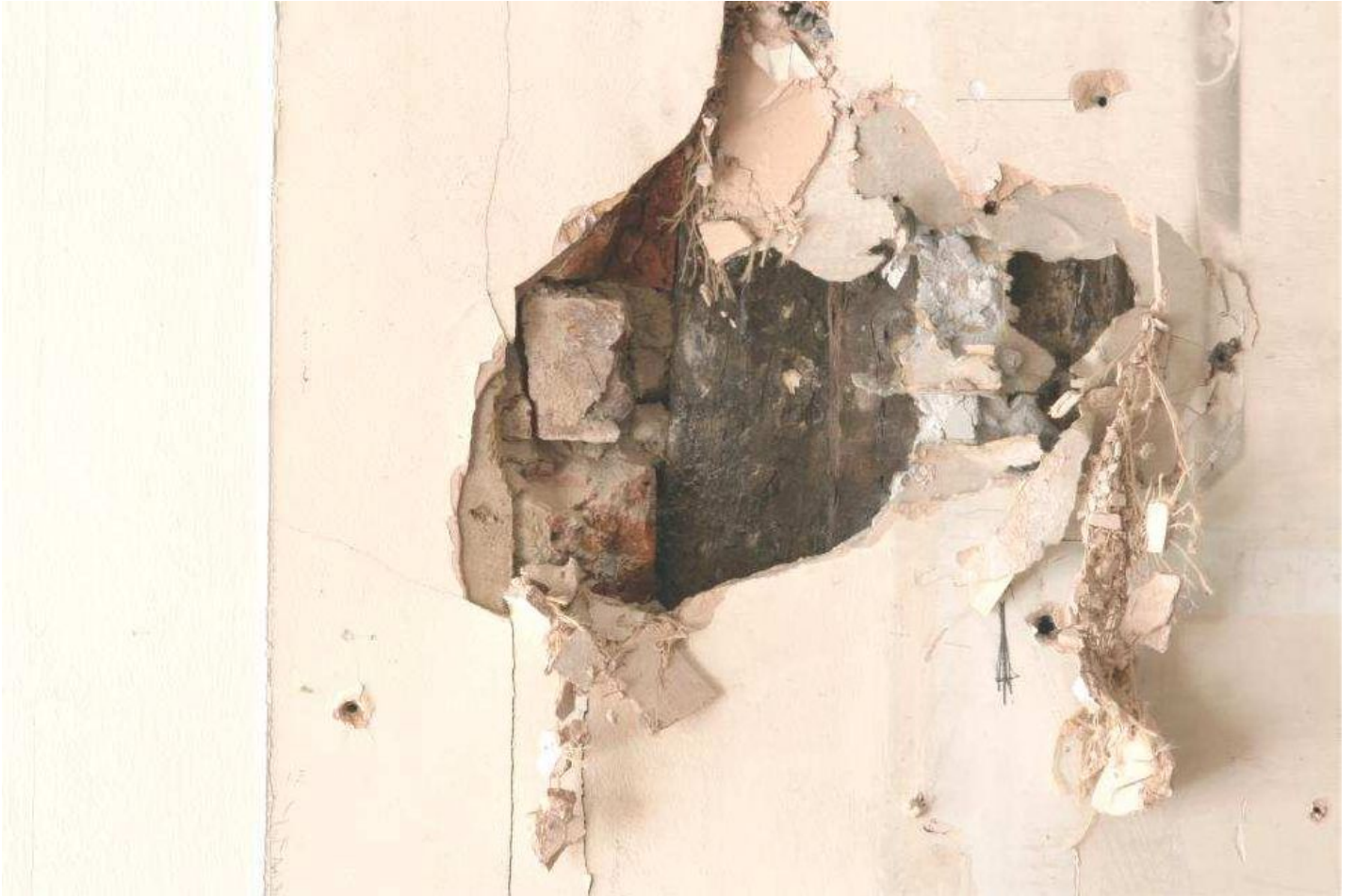
Plate 03 - Test-hole in plaster showing studwork behind
