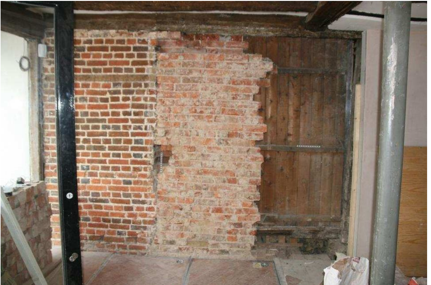
Plate 06 - Blocked opening in E elevation of No2
