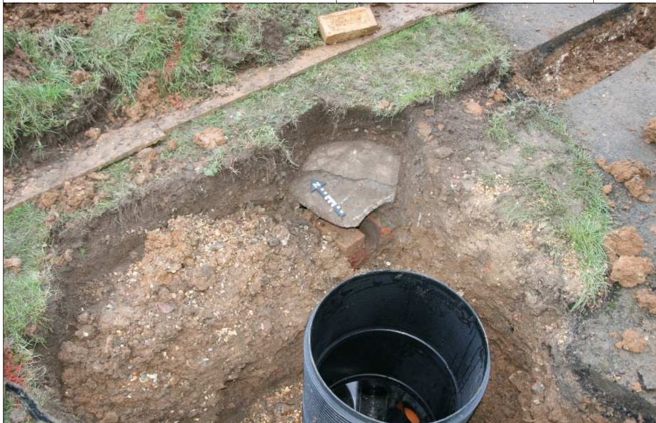
Plate 10: Buried grave slab in manhole pit
