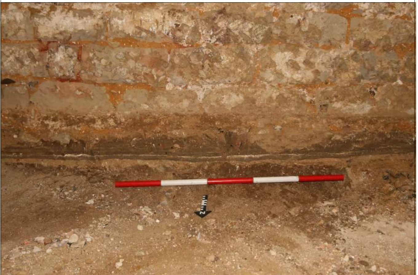
Plate 12: South wall of west tower, section below the stonework at the east end
