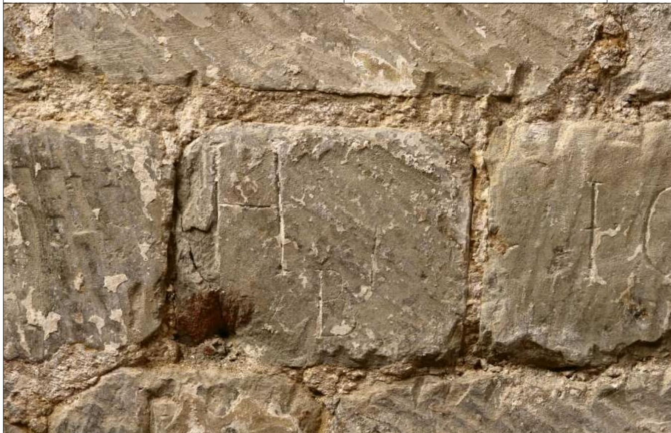
Plate 41: Detail of graffiti on N wall of tower, letters H B I
