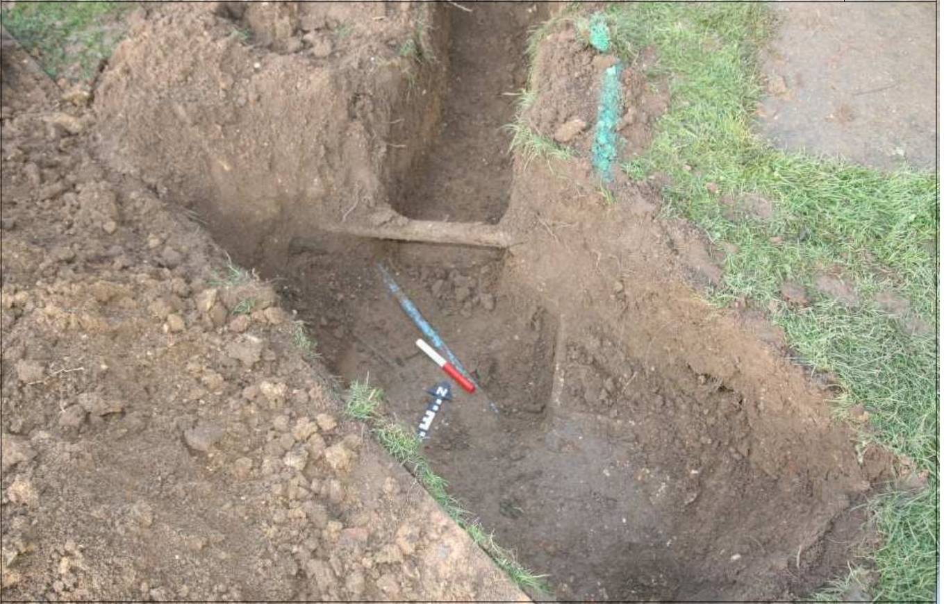
Plate 7: Trial pit 3, showing the existing watermain, electric cables and S end of Tr.3
