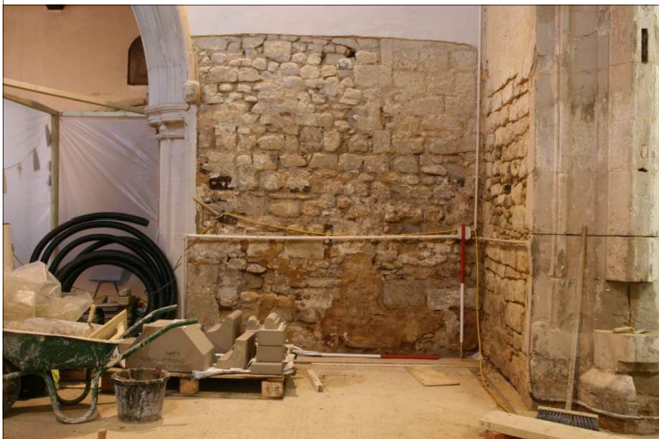
Plate 32: West end of the southern nave wall , showing blocked opening, looking S
