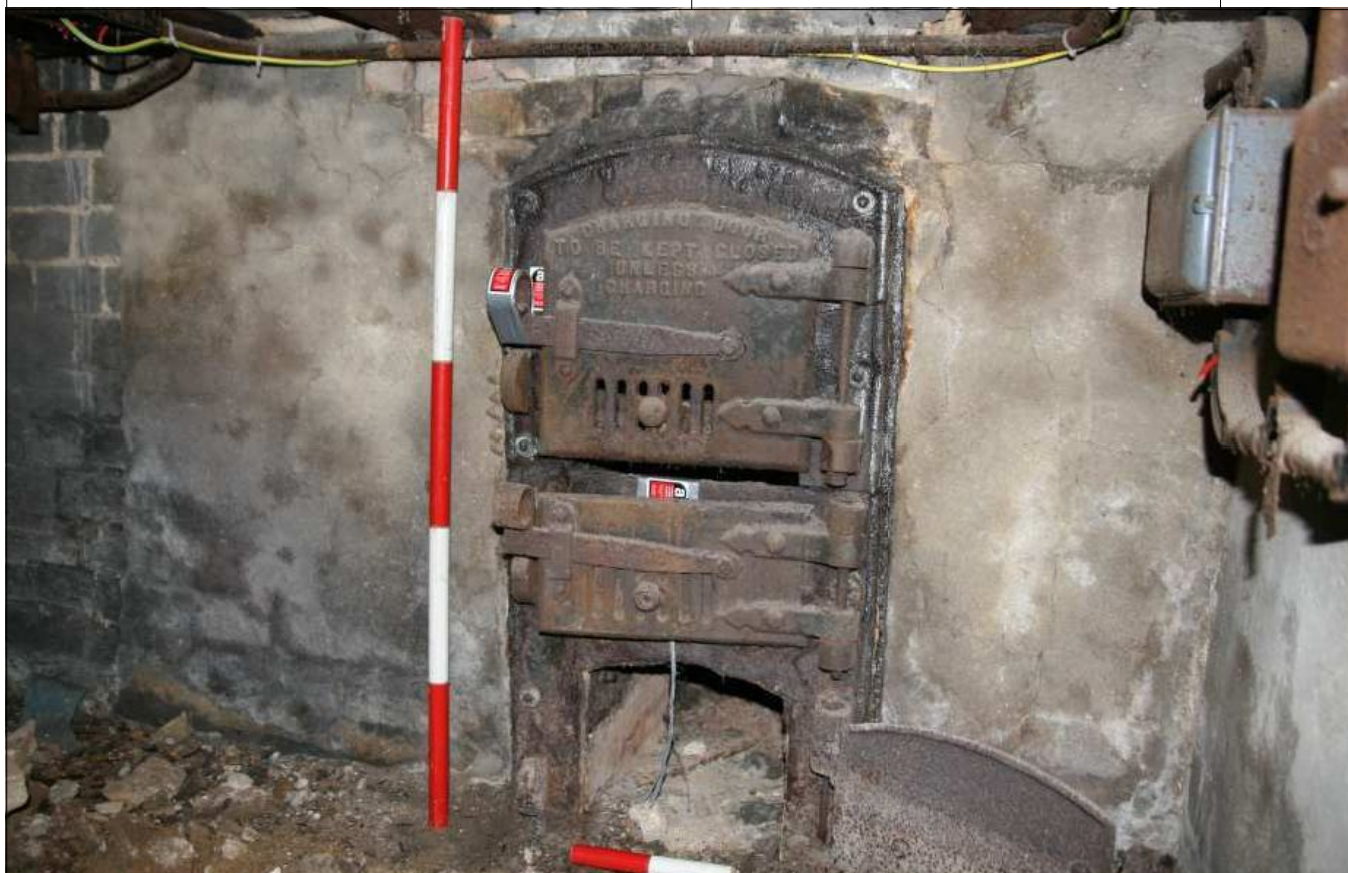
Plate 19: Front of boiler in E elevation of structure [2], looking E
