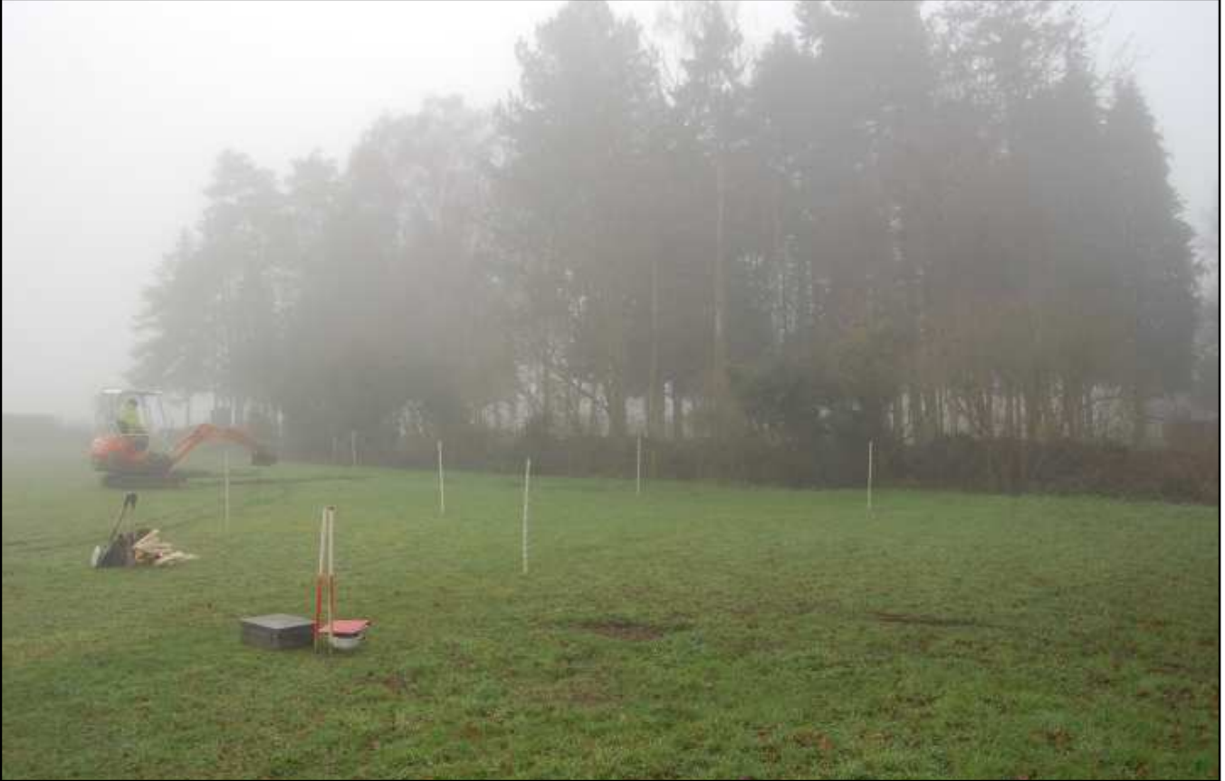
Plate 1: General view across the site prior to the start of the groundworks, looking SW
