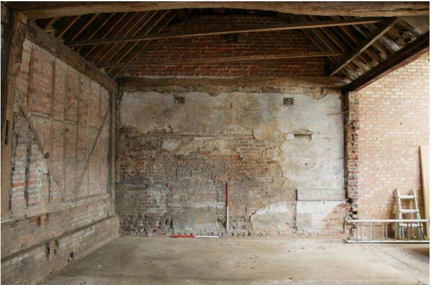
Plate 20 - South-west interior elevation after removal of plaster (c) The Heritage Network Ltd.
