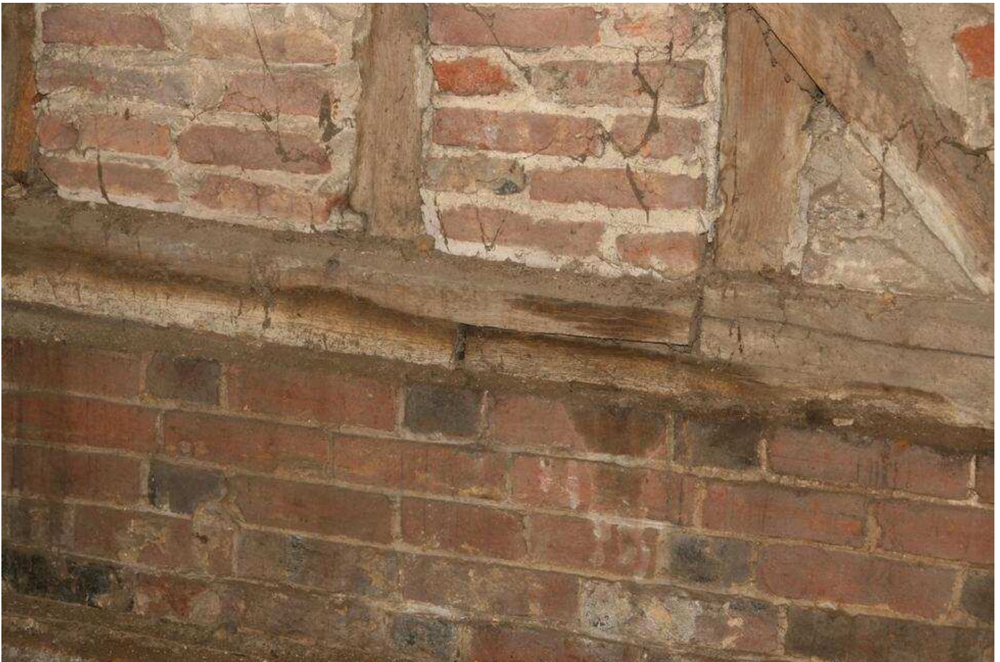
Plate 18 - Detail of butt joint in sole plate, Bay 3 (c) The Heritage Network Ltd.
