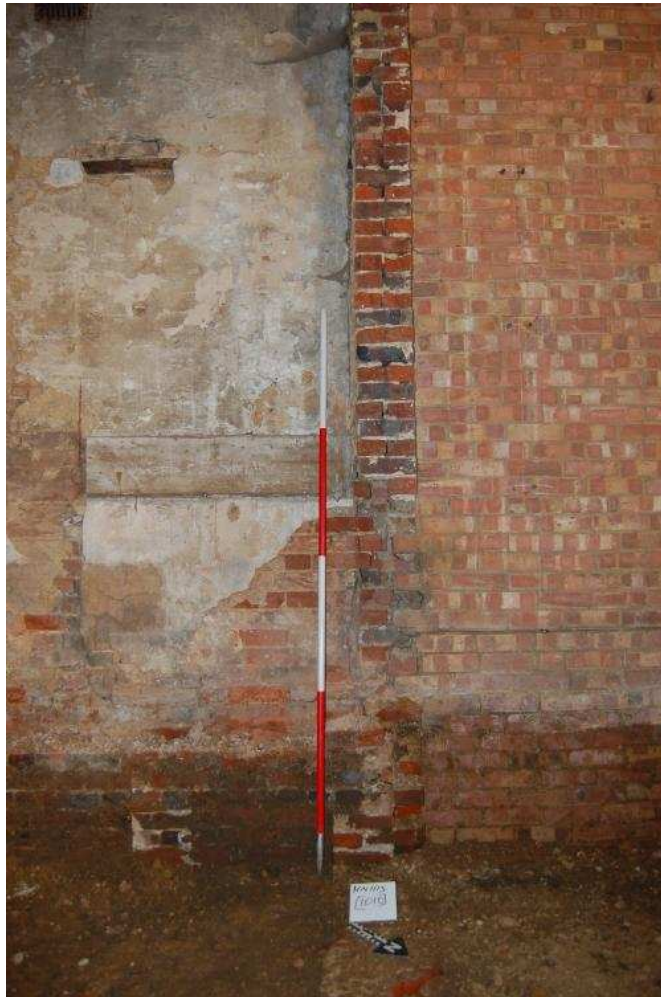
Plate 21 - Blocked opening in SW elevation
