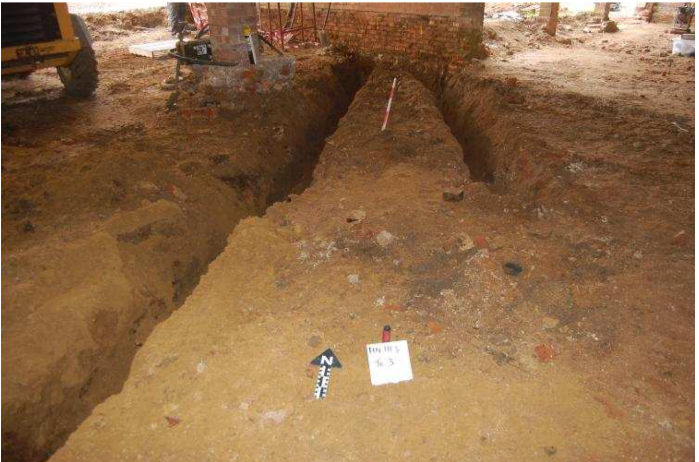
Plate 42 - Service trenches at SW end of barn, looking N (c) The Heritage Network Ltd.
