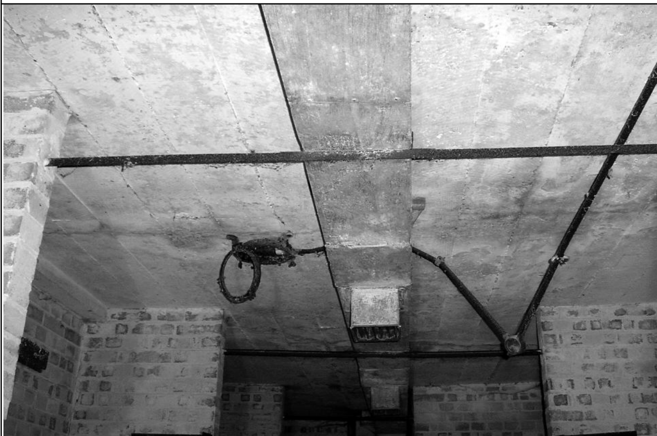
Plate 16: Area 11, eastern sleeping shelter, detail of air duct and electrical trunking
