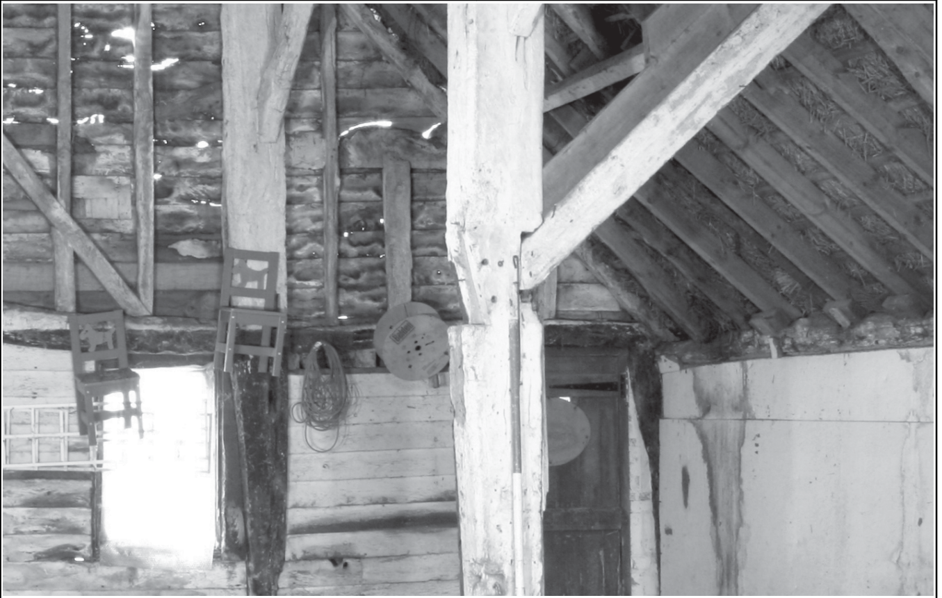
Plate 11: Integral bracket in second arcade post from the north
