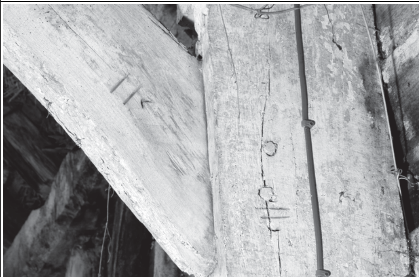
Plate 8: Carpenter's marks on northern face of the second frame from the north
