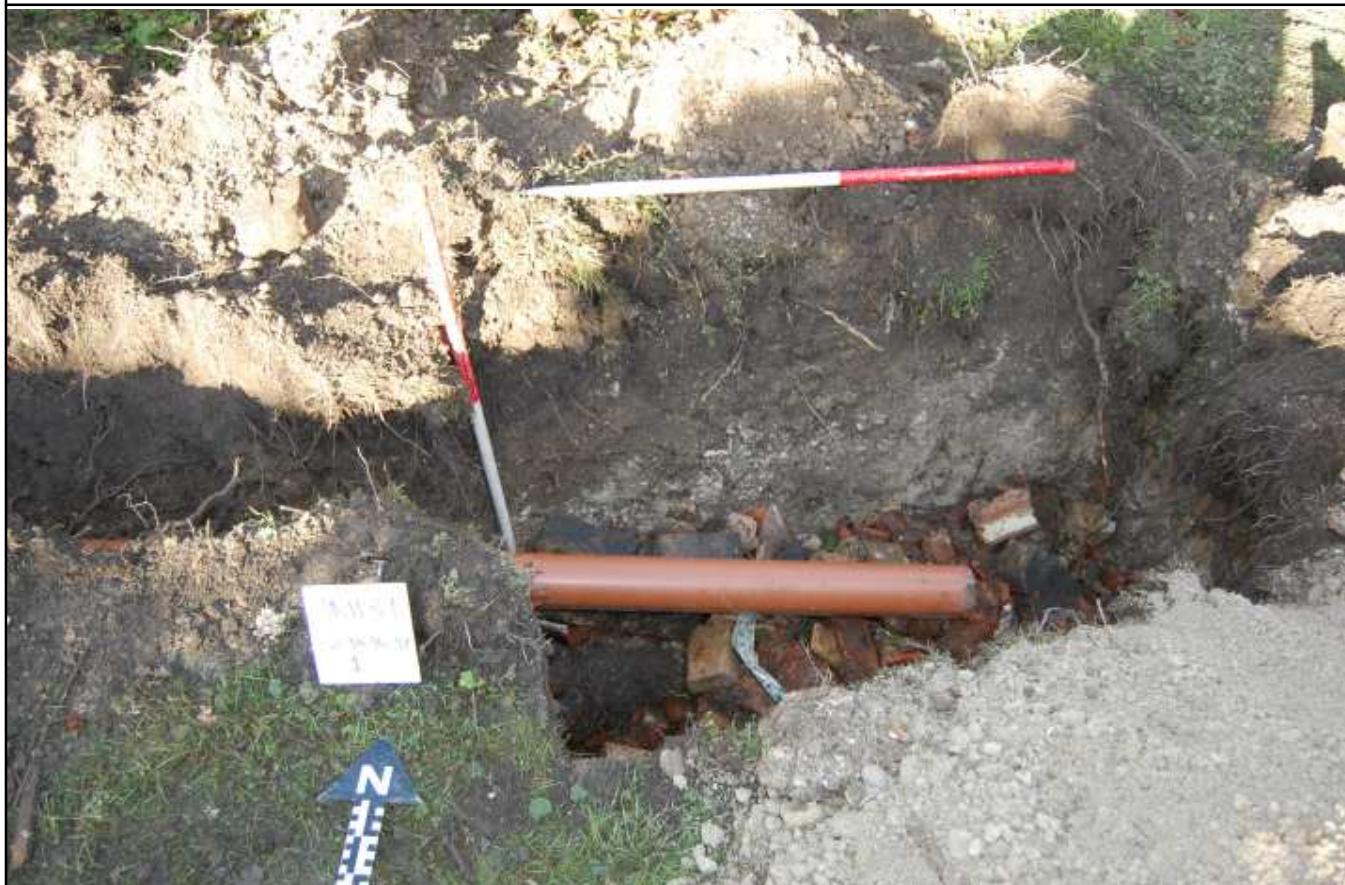
Plate 12: Soakaway, looking N
