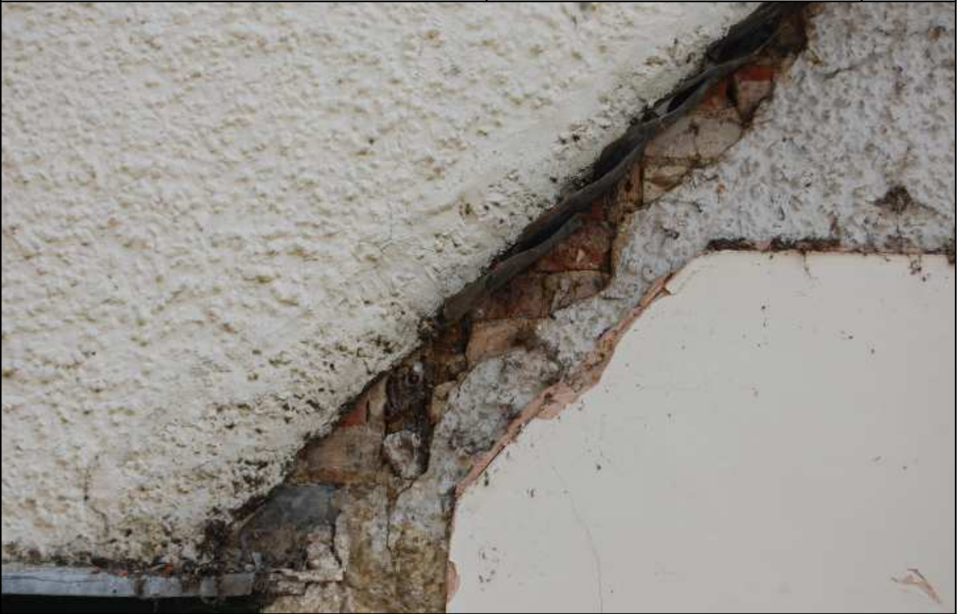
Plate 5: Narrow strip of brickwork exposed below the render, S end of north block
