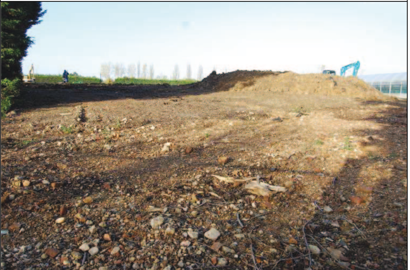
Plate 2: Overburden height from original ground level; East end of site, looking south.
