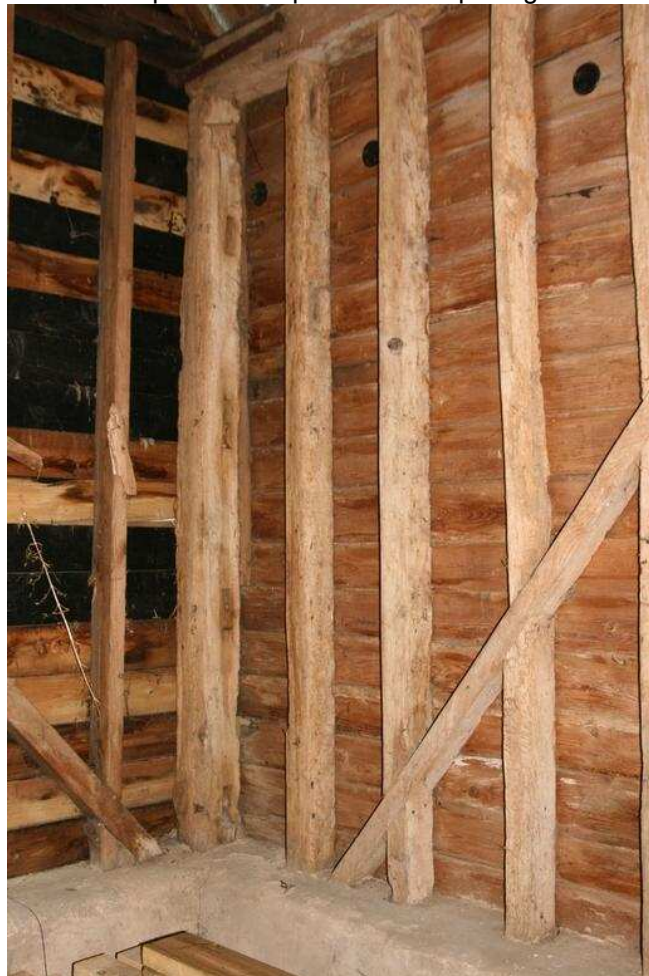
Plate 18 - Bay 1, NE elevation, showing weathered studs
