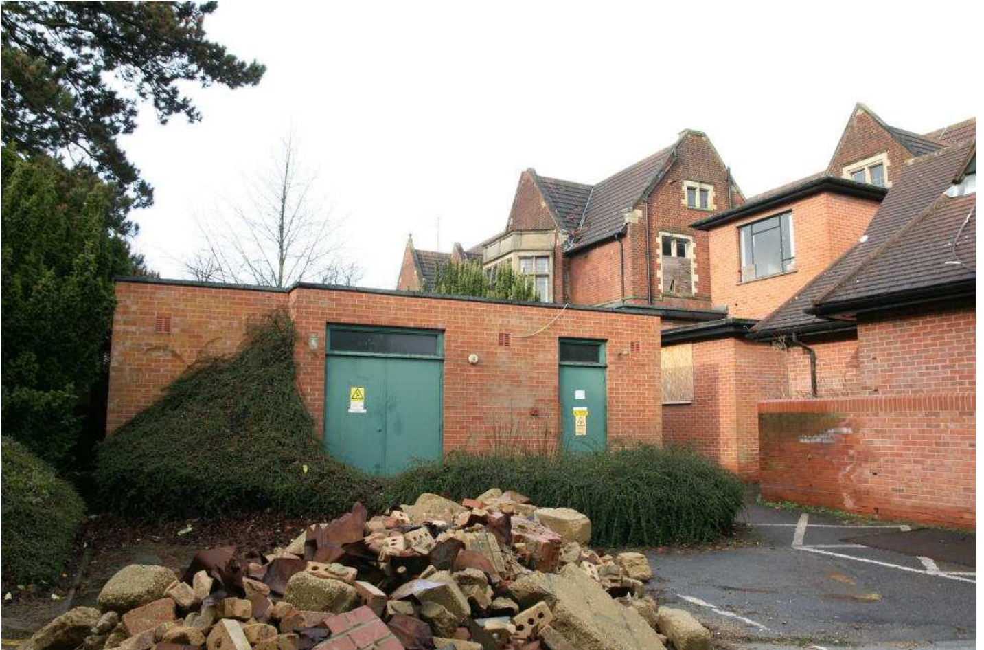
Plate 01 - Electricity sub-station, facing north-west
