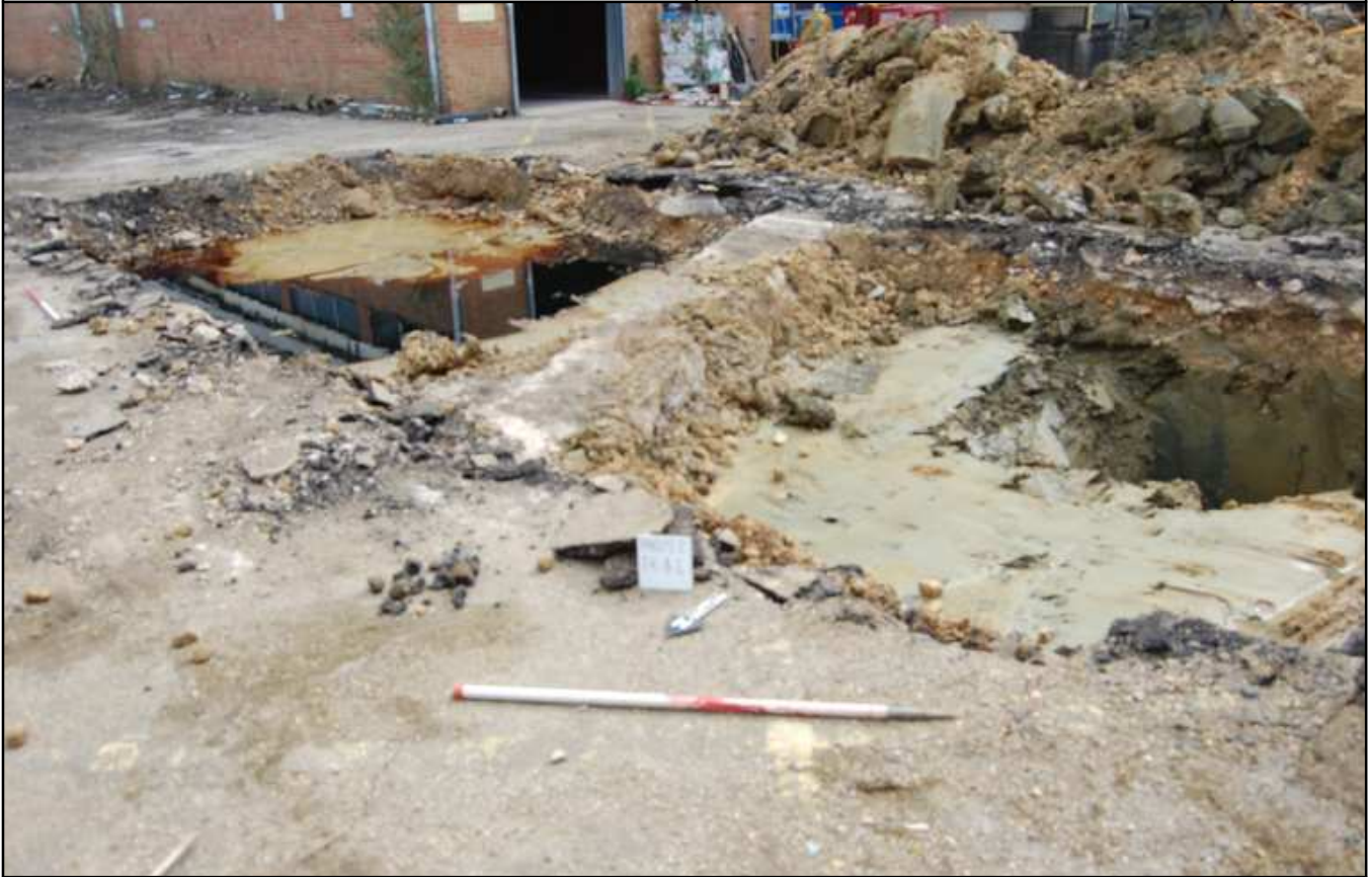
Plate B1: Trench B1, showing contaminated ground, looking southeast
