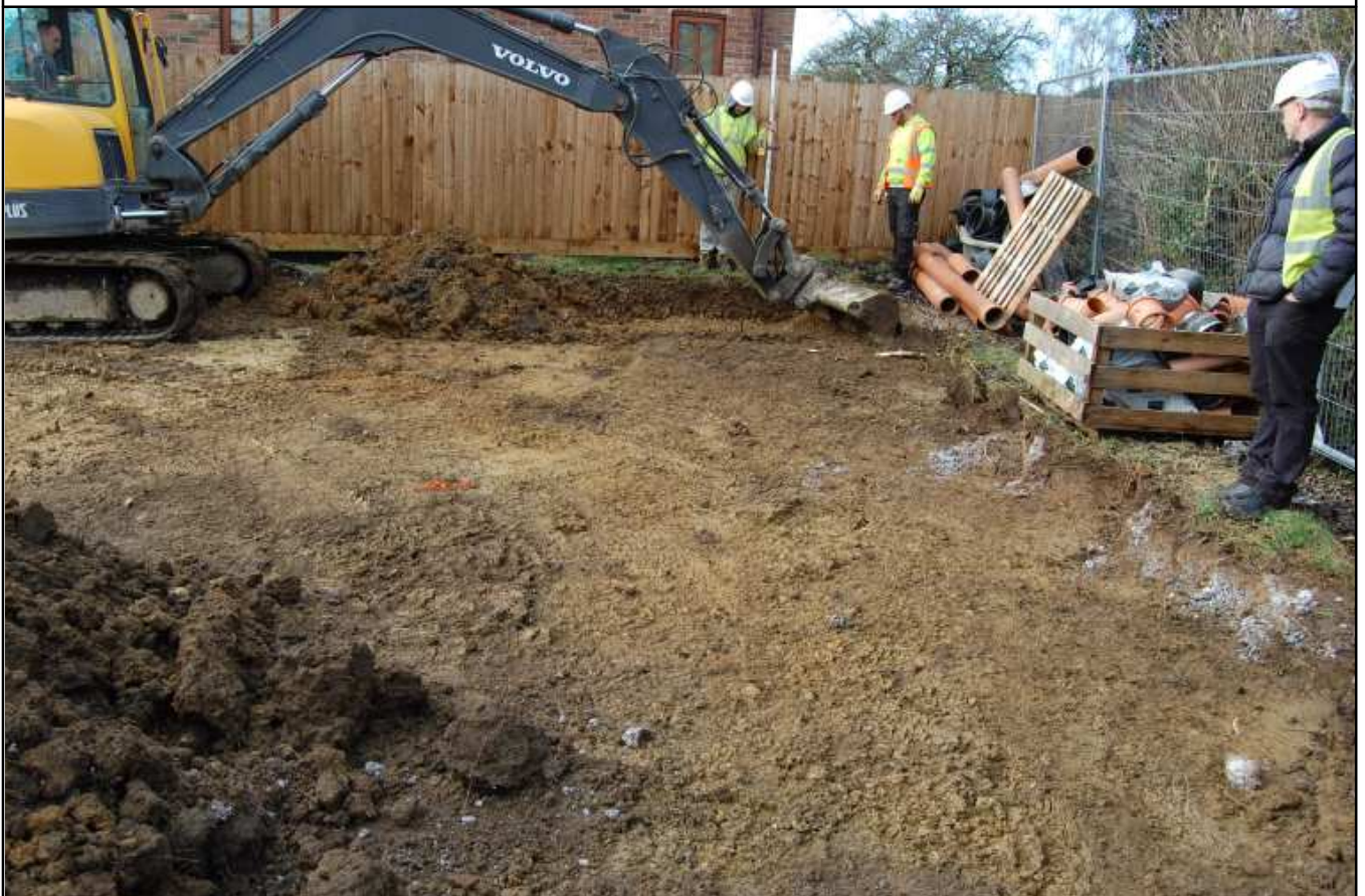
Plate 2: Working shot showing clay natural and modern soakaway in centre of shot, looking west
