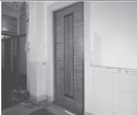
Frame 7: Admin Block, 1st floor N door to board room, facing NE
