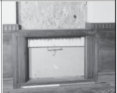
Frame 9: Canteen Managers' dining room, rad. enclosure
