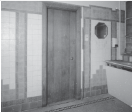
Frame 8: Admin Block, G floor WC adj. Room 32, S cubicle, facing S
