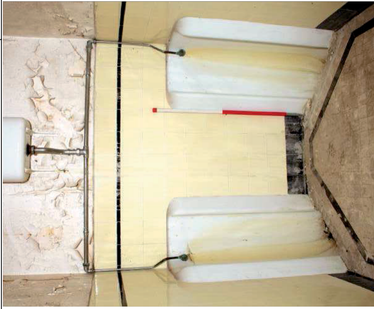
Plate 46: Canteen block, ground floor, gent's lavatory adjacent to N entrance (Full report, para.3.7)
