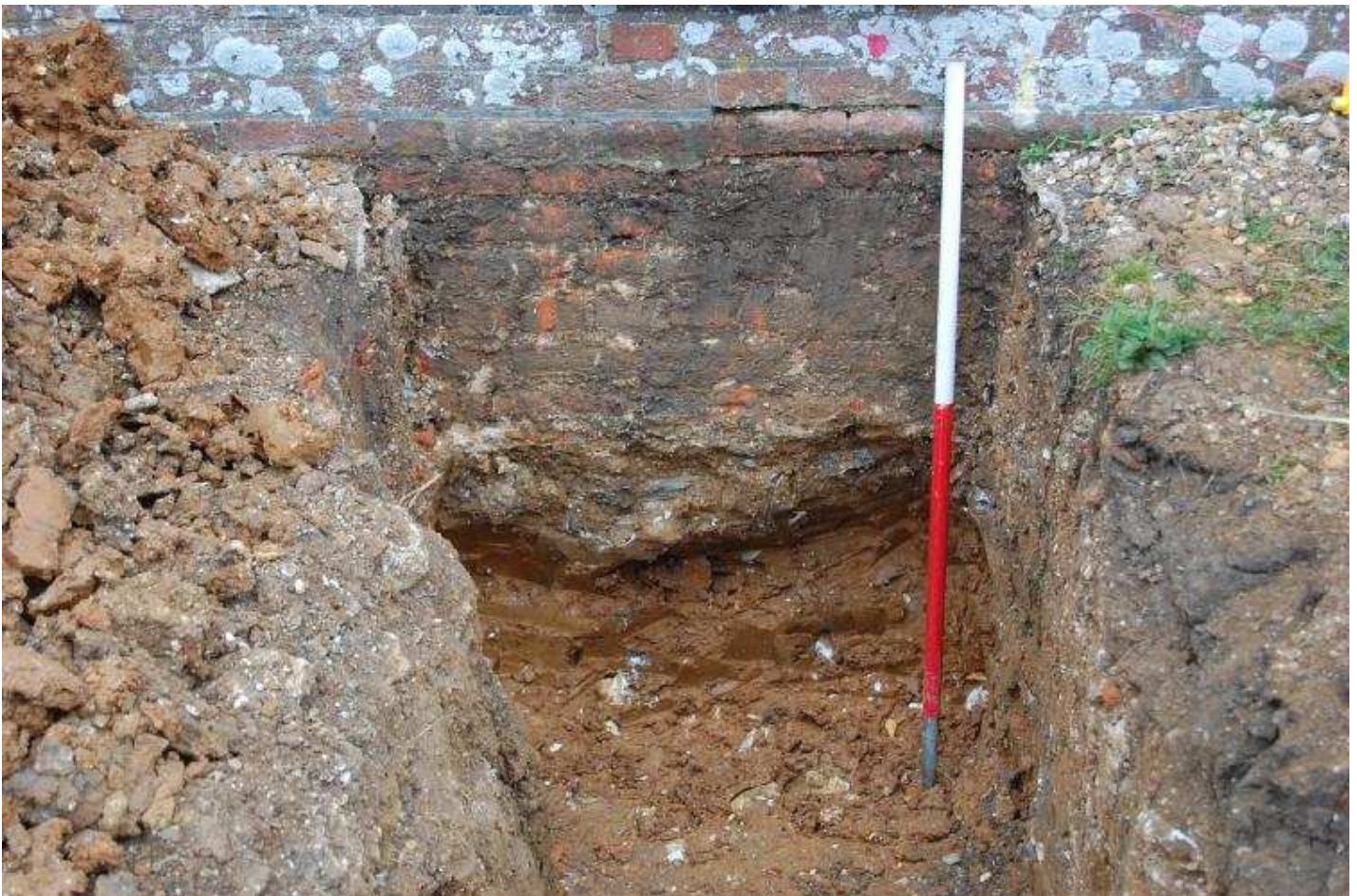
Plate 006 - Footings trench, showing earlier foundation [102], looking N (c) The Heritage Network Ltd.
