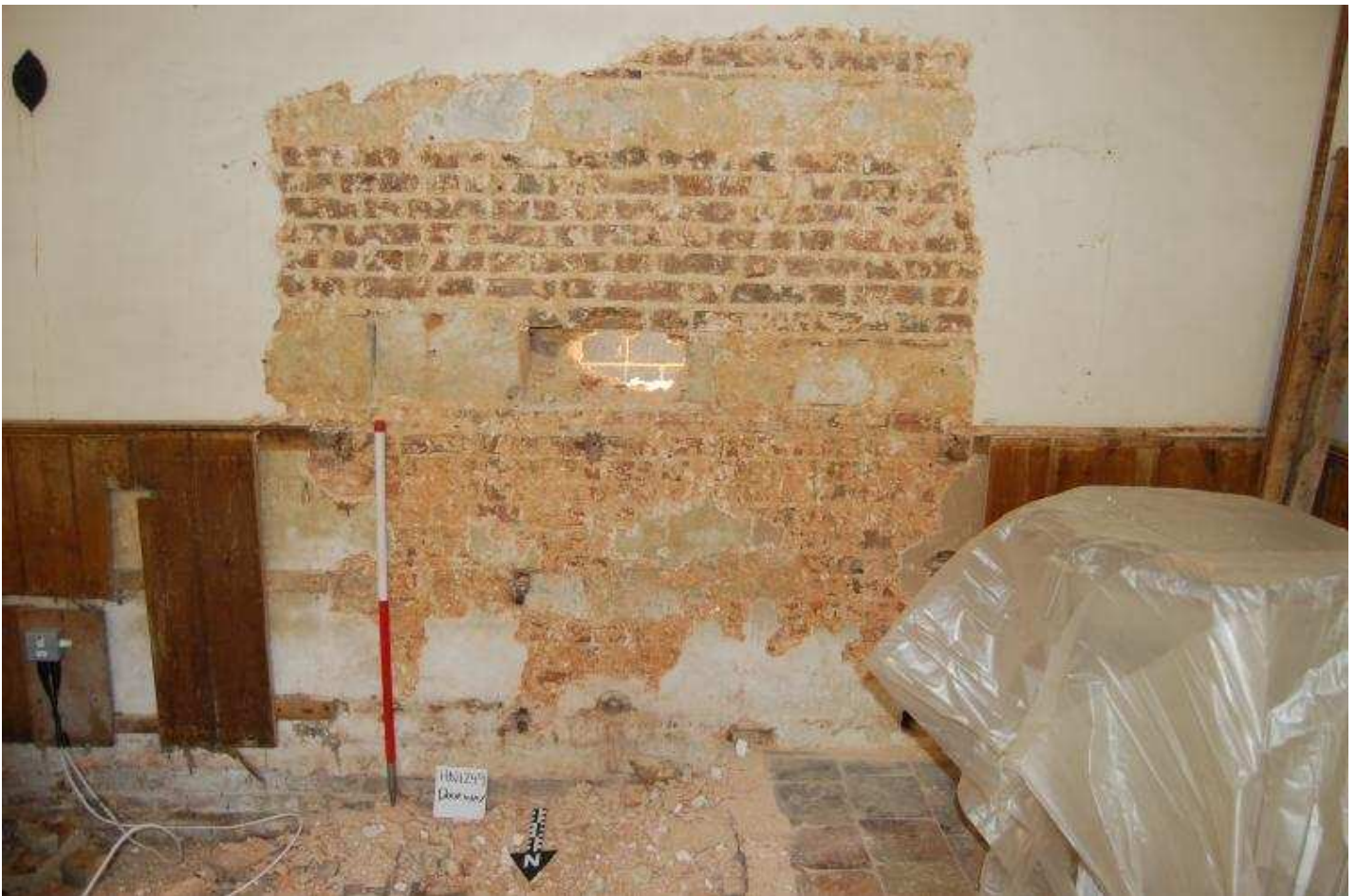
Plate 018 - S wall of nave after removal of plaster (c) The Heritage Network Ltd.
