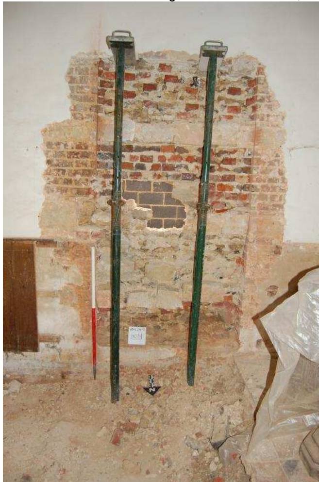
Plate 020 - New doorway after removal of interior brick facing (c) The Heritage Network Ltd.
