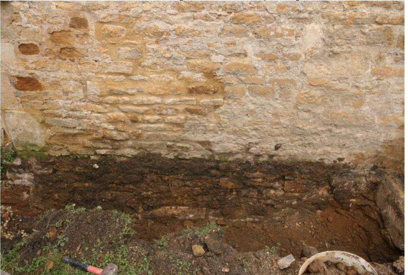
Plate 04 - Footings to N wall of church, looking S (c) The Heritage Network Ltd.
