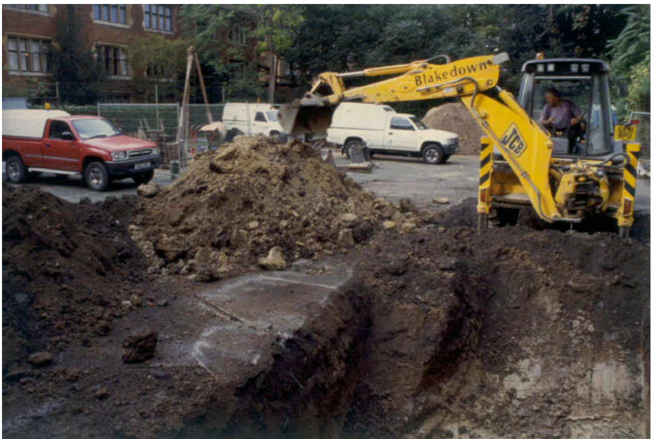
Fig 14: General view looking north-west across the site, showing the JCB opening trench 2, with the geotechnical bore-hole rig to left, and with the spoil heap from trench 1 in the background. Buildings on Church Close stand beyond the site
