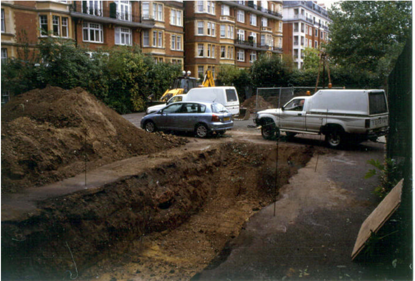
Fig 13: View looking south-east across the site during initial machining work, with trench 1 in the foreground and with the JCB in the background working on opening trench 2. The legs of the geotechnical bore-hole rig can be seen to the right. York House stands beyond the site
