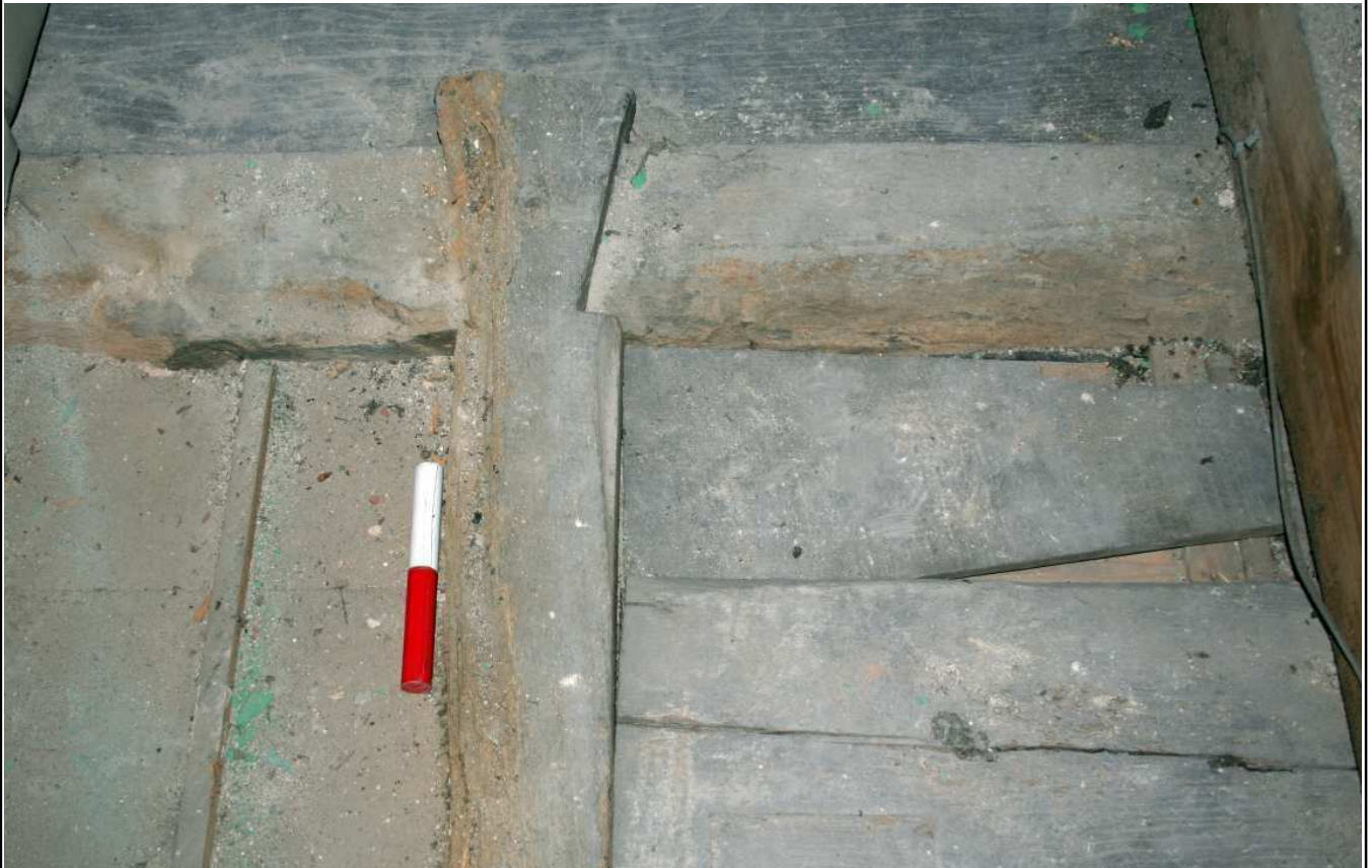
Plate 41: Attic, detail of dovetail joint between central joist and brace to wall plate
