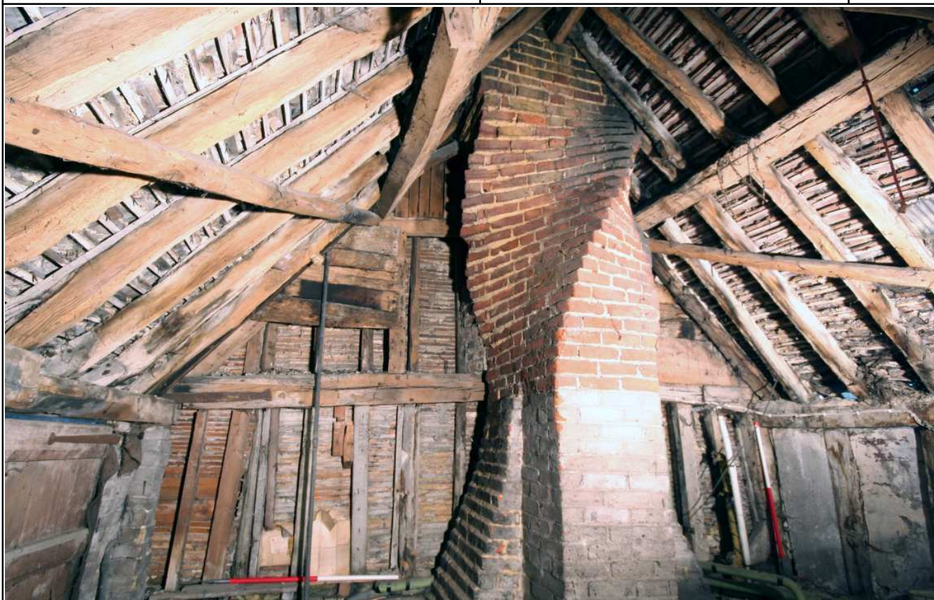
Plate 67: Rear range, 1st floor, Bay 1, twisted chimney looking west
