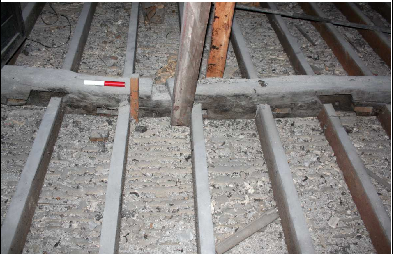
Plate 42: Attic, detail of mortice for missing brace to eastern wall plate
