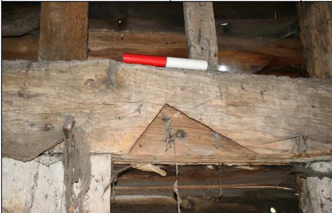
Plate 17: Upper floor, detail of cut-out for lapped timber in southern tie beam
