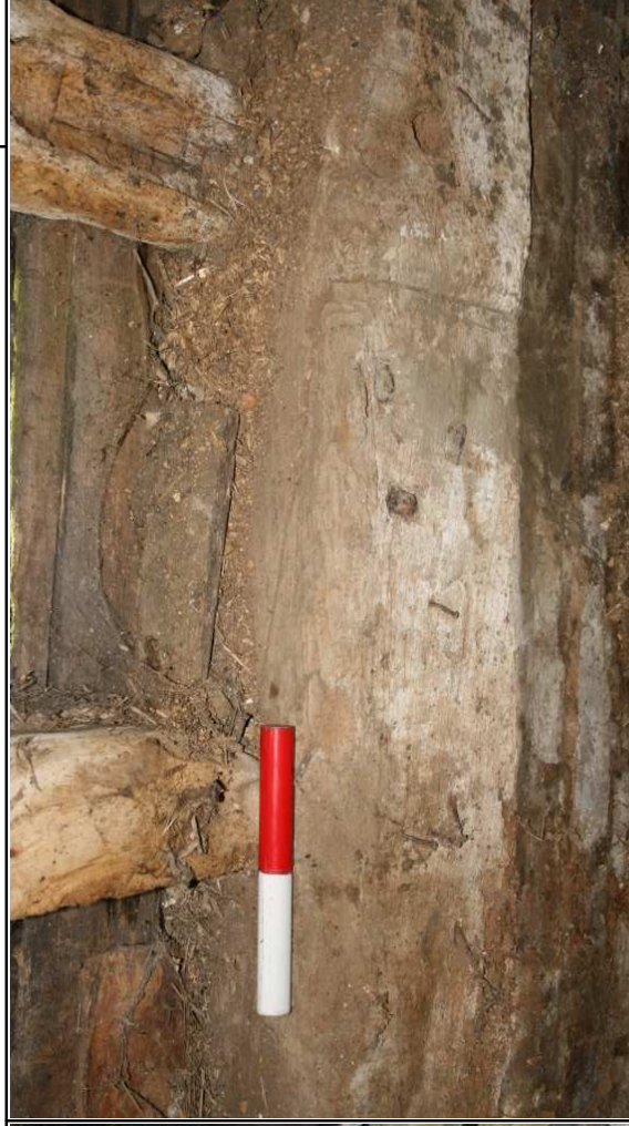
Plate 10: North Barn, N elevation Bay 2, face halved & bladed joint in sill beam
