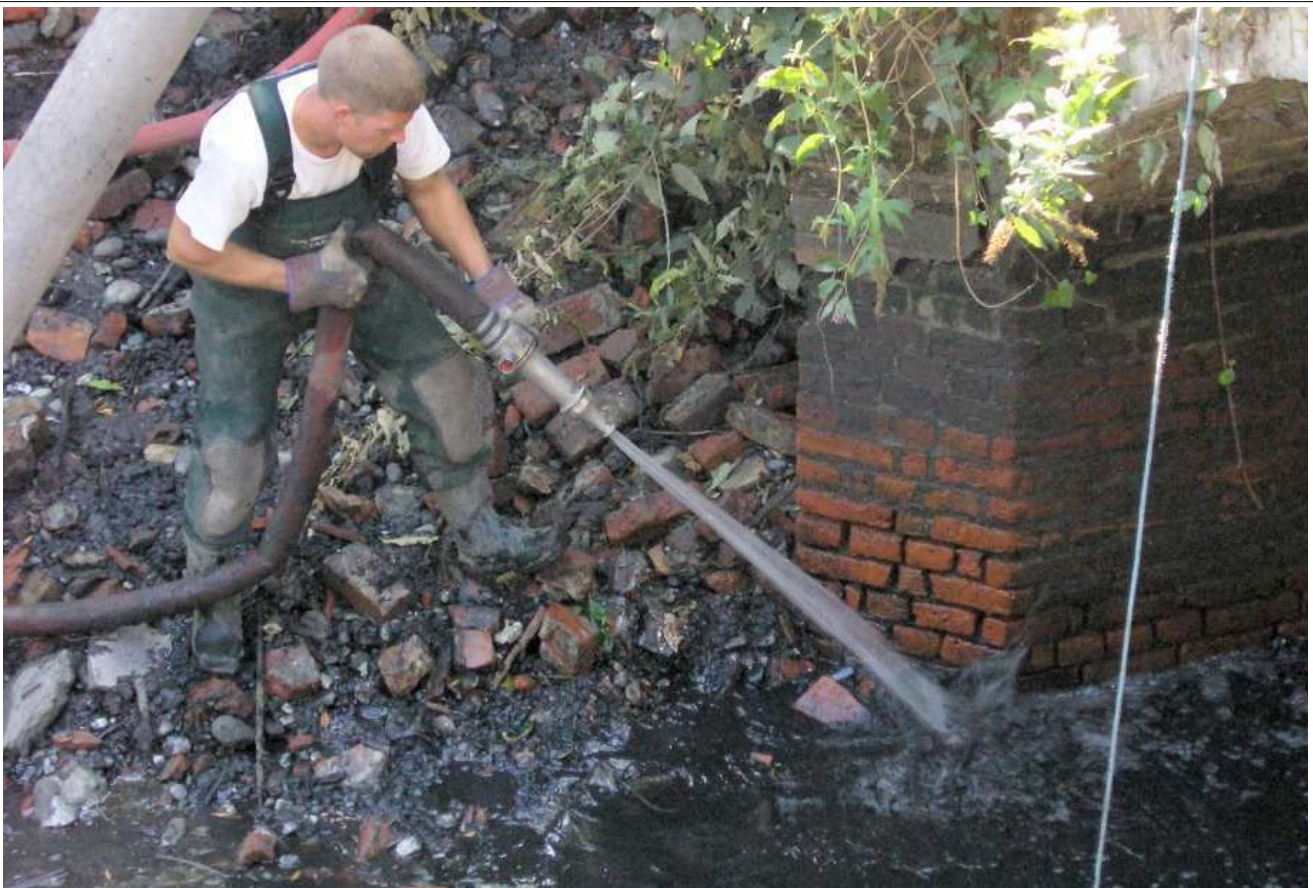
Plate 6: Using a water-jet to clear silts from around the SW bridge pier
