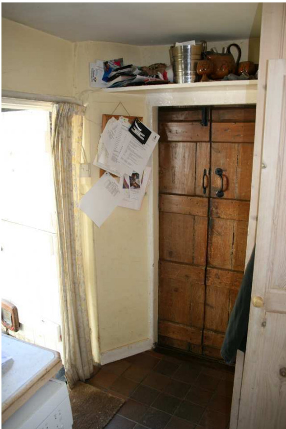
Plate 11: Cottage, S elevation of kitchen, E end, showing door cut through wall, looking S
