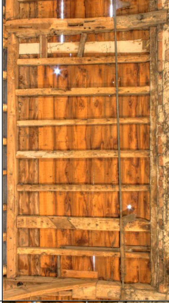
Plate 28: Barn: S elevation, Bay 3, showing mixture of modern & re-used timbers in framing
