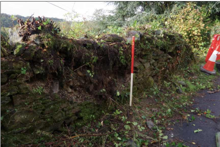
Plate 2: Pre-commencement view of retaining wall parapet showing collapse of the face (left of scale) and surviving capping (right). Looking southwest (scale 1m)
