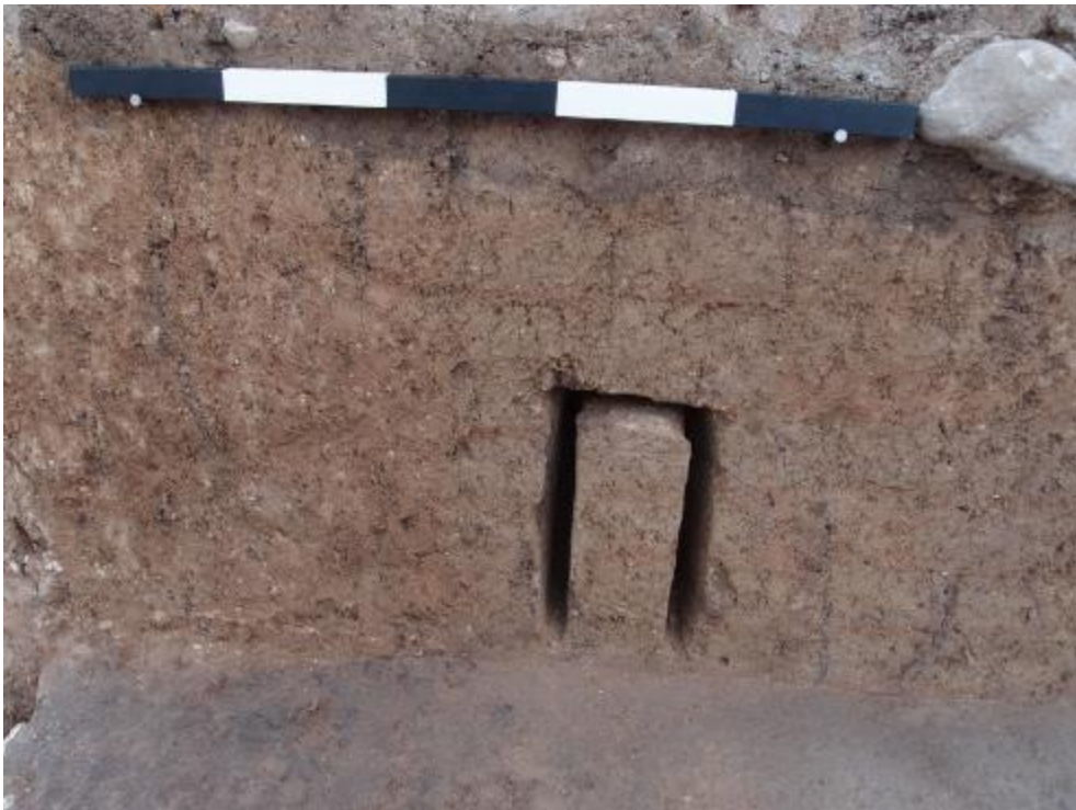
Figure 3.3. Mud brick wall (W64) with green mudbricks and slightly reddish brown mortar, Trench 10 (SW).
