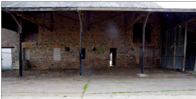
Plate 6: West end of north elevation of north barn, looking south (1m scale)
