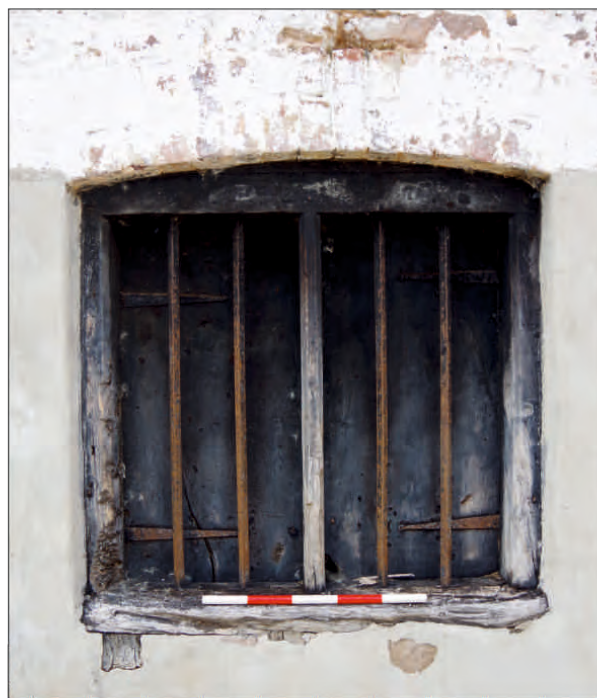
Plate 17: Ground-floor window in the east elevation of the west barn, looking west (0.50m scale)
