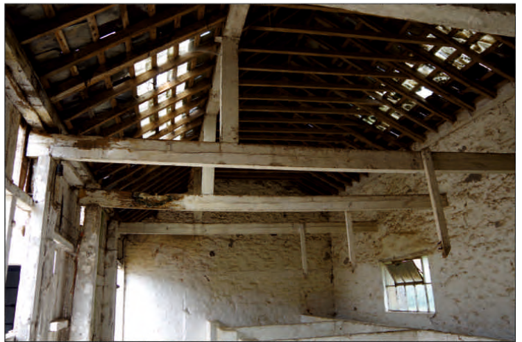
Plate 26: Roof structure in north end of ground floor of east barn, looking north (1m scale)
