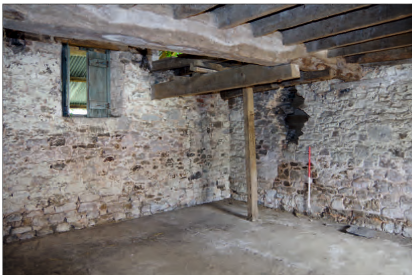
Plate 21: General view of north room on the ground floor of the west barn, looking northwest (1m scale)
