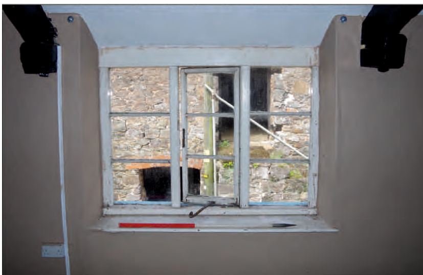
Plate 12: Three-light window in the west end of the south barn, looking north (1m scale)
