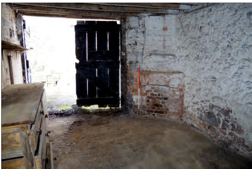
Plate 15: General view of tool house on the ground floor of the south barn, looking northeast (1m scale)
