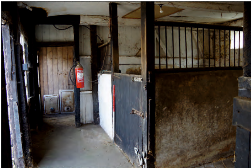
Plate 14: General view of stables on the ground floor of the south barn, looking east (1m scale)
